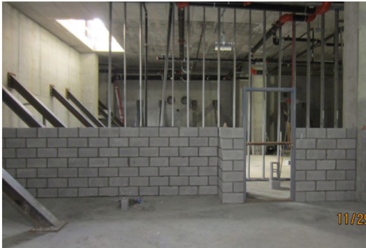
Hilton Cleveland Downtown, Cleveland, Ohio Contract Number: 140177 Photo 161 - B1 Level Masonry Date: November 29, 2014
