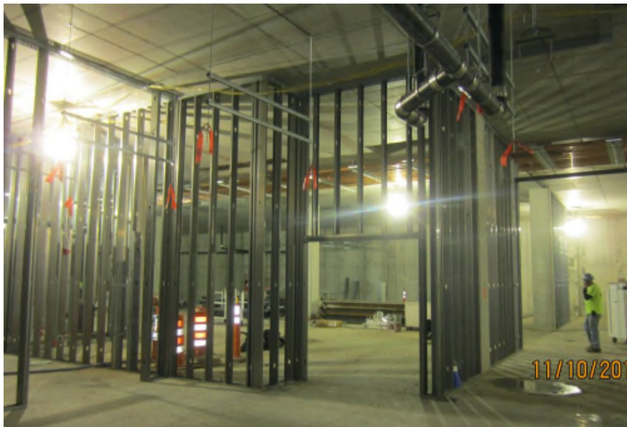
Hilton Cleveland Downtown, Cleveland, Ohio Contract Number: 140177 Photo 153 - Main Electrical Room Framing Date: November 10, 2014
