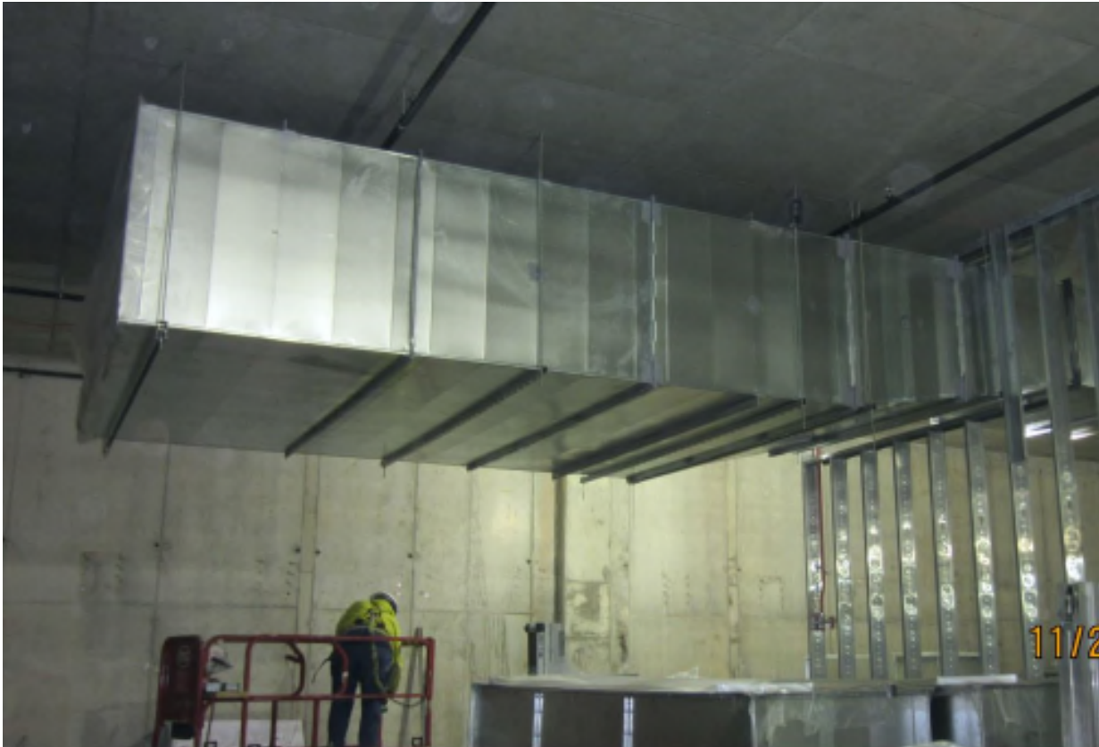
Hilton Cleveland Downtown, Cleveland, Ohio Contract Number: 140177 Photo 156 - B1 Level Ductwork Date: November 20, 2014
