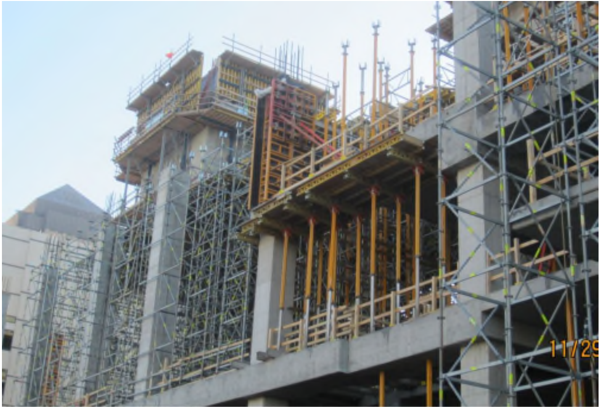
Hilton Cleveland Downtown, Cleveland, Ohio Contract Number: 140177 Photo 163 - 5th Floor High Shoring Date: November 28, 2014
