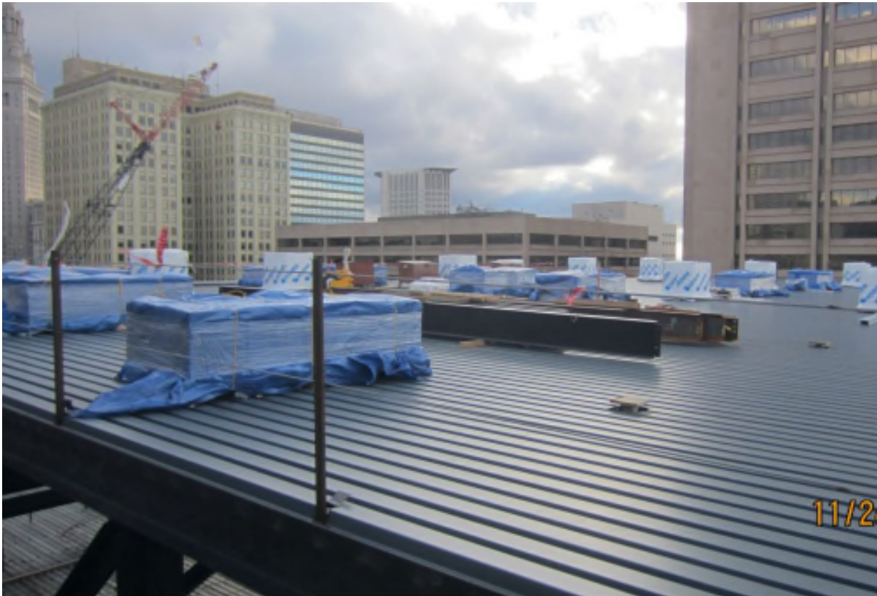
Hilton Cleveland Downtown, Cleveland, Ohio Contract Number: 140177 Photo 159 - Podium Roof Deck / Material Date: November 24, 2014
