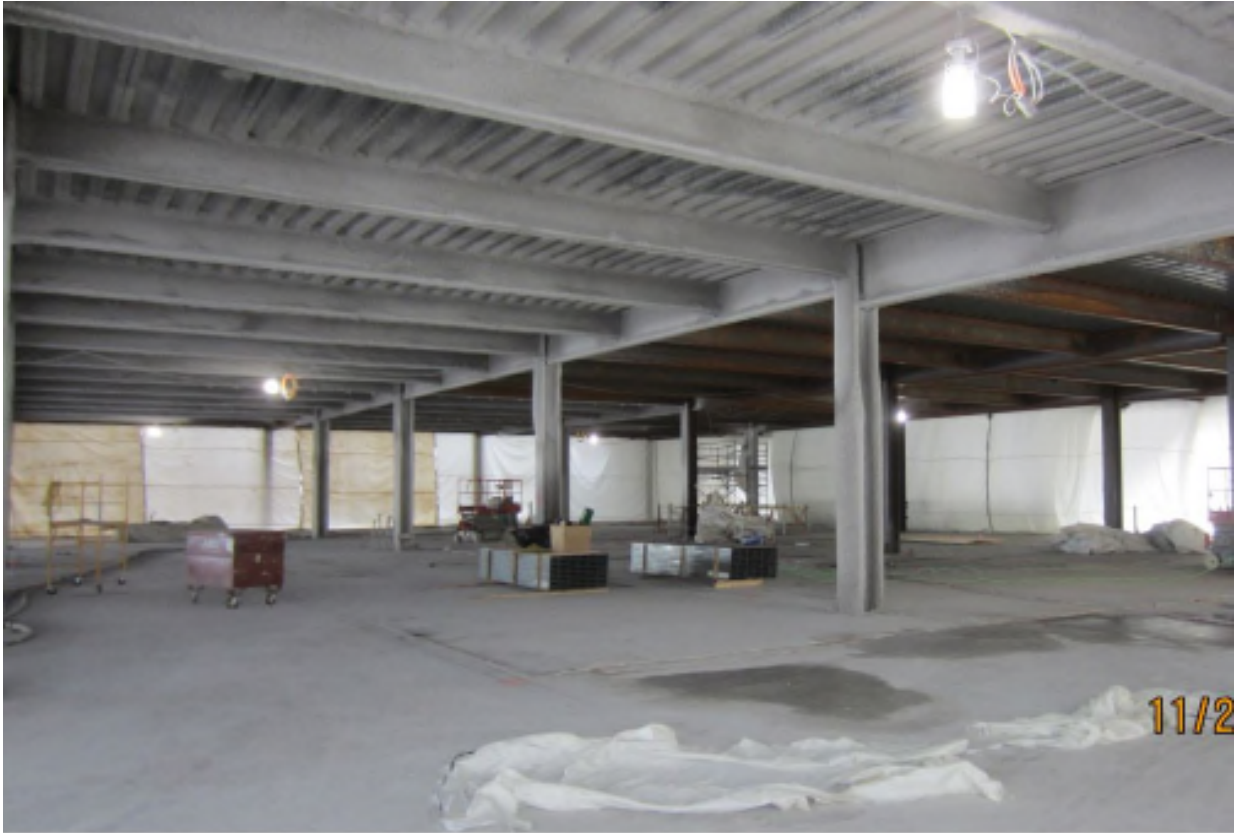
Hilton Cleveland Downtown, Cleveland, Ohio Contract Number: 140177 Photo 162 - 2nd Floor Spray-on Fireproofing Date: November 28, 2014
