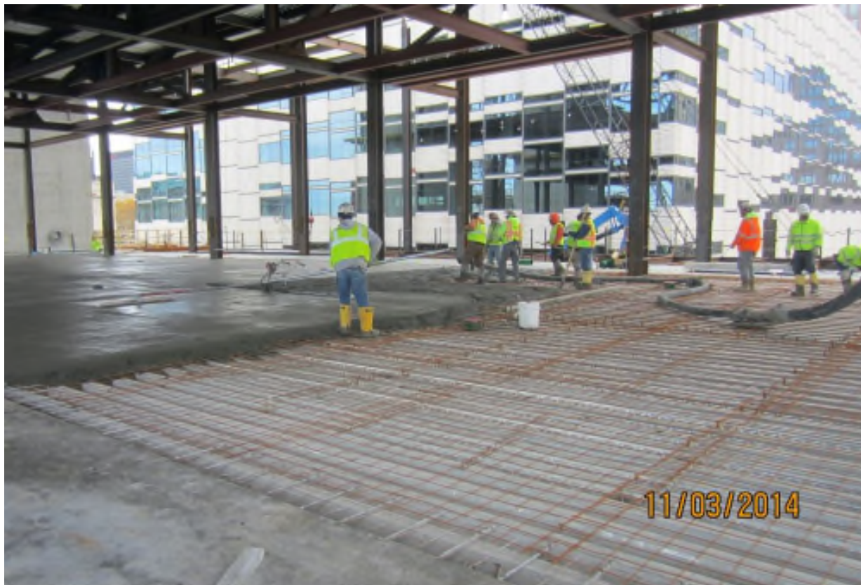
Hilton Cleveland Downtown, Cleveland, Ohio Contract Number: 140177 Photo 152 - 3rd Floor Slab-on-metal-deck Date: November 3, 2014
