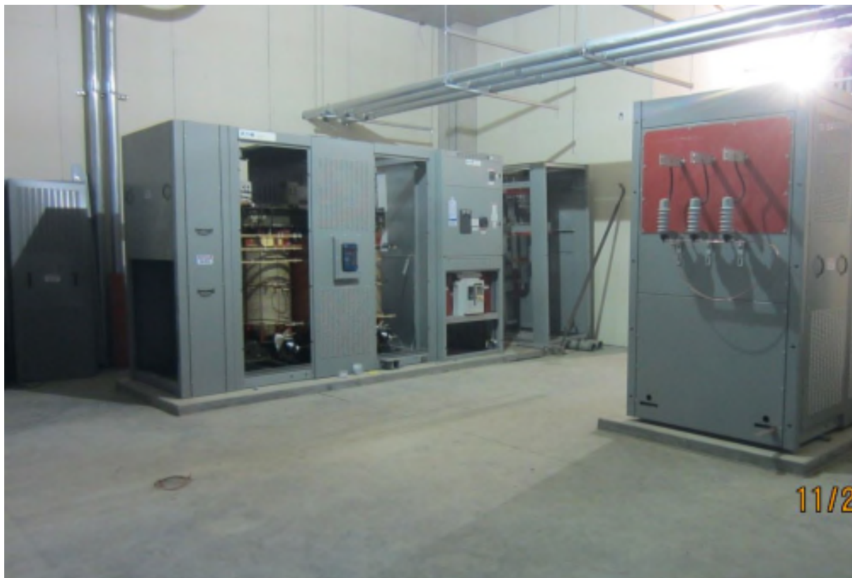
Hilton Cleveland Downtown, Cleveland, Ohio Contract Number: 140177 Photo 160 - B1 Electrical Switchgear Date: November 25, 2014
