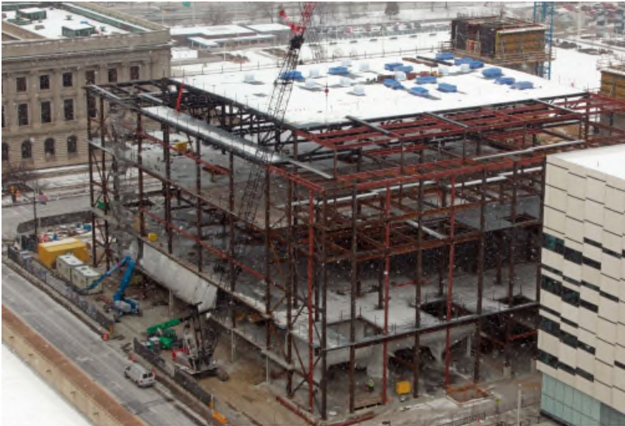
Hilton Cleveland Downtown, Cleveland, Ohio Contract Number: 140177 Photo 158 - Project Progress Date: November 21, 2014
