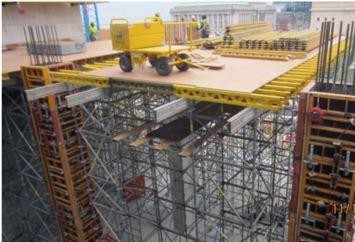
Hilton Cleveland Downtown, Cleveland, Ohio Contract Number: 140177 Photo 154 - 5th Floor Concrete Formwork Date: November 12, 2014
