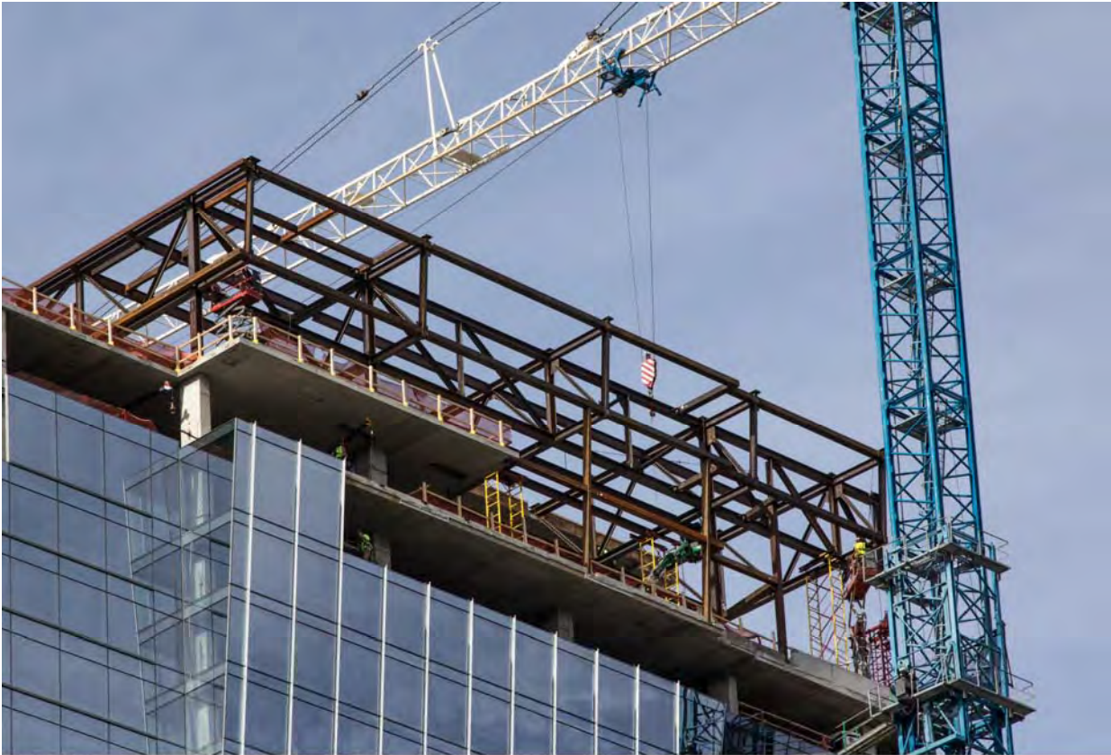
Hilton Cleveland Downtown, Cleveland, Ohio Contract Number: 140177 Photo 301 - Top-of-tower Steel Date: September 25, 2015
