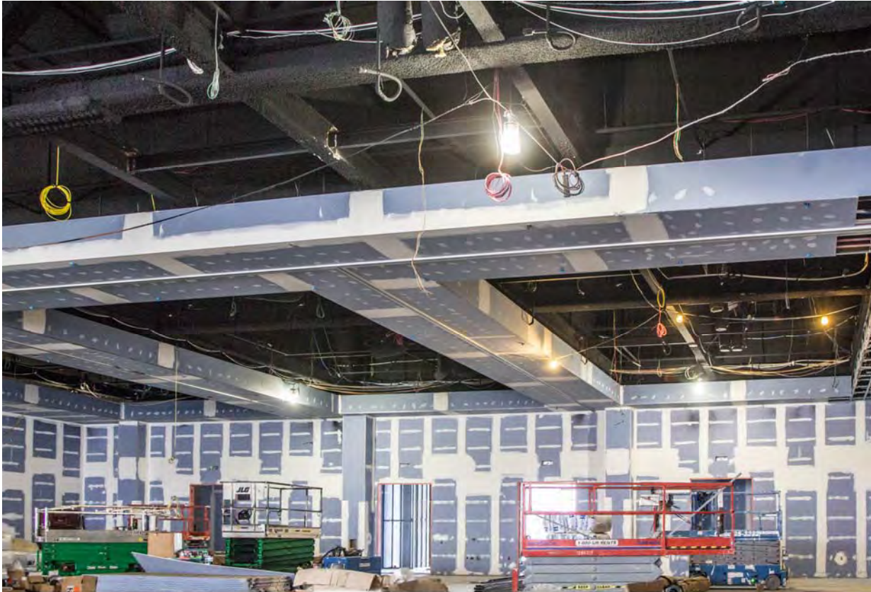
Hilton Cleveland Downtown, Cleveland, Ohio Contract Number: 140177 Photo 303 - 3rd Floor Jr. Ballroom Date: September 28, 2015
