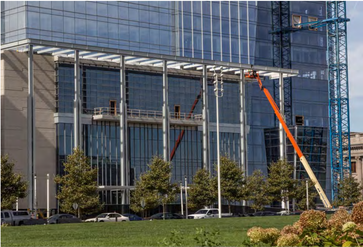
Hilton Cleveland Downtown, Cleveland, Ohio Contract Number: 140177 Photo 302 - East Elevation at West Mall Drive Date: September 25, 2015
