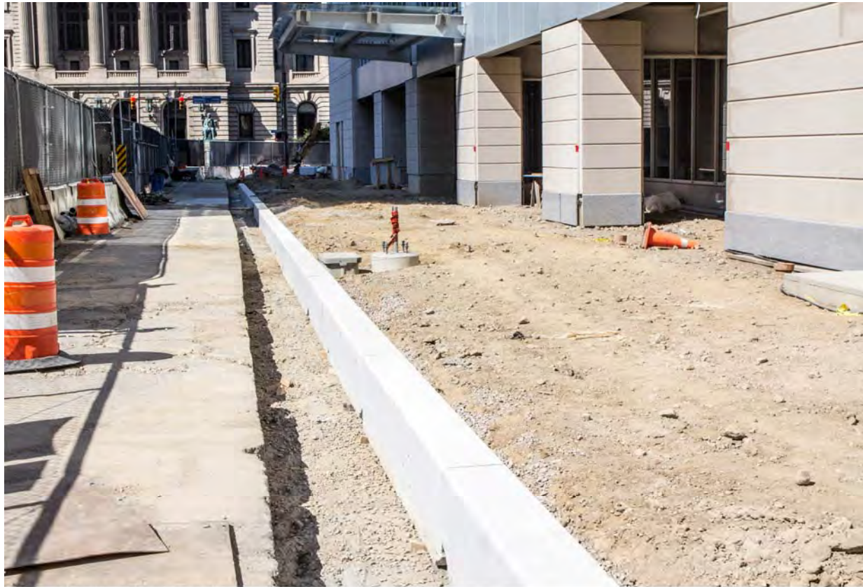
Hilton Cleveland Downtown, Cleveland, Ohio Contract Number: 140177 Photo 297 - Ontario Street Granite Curbs Date: September 17, 2015
