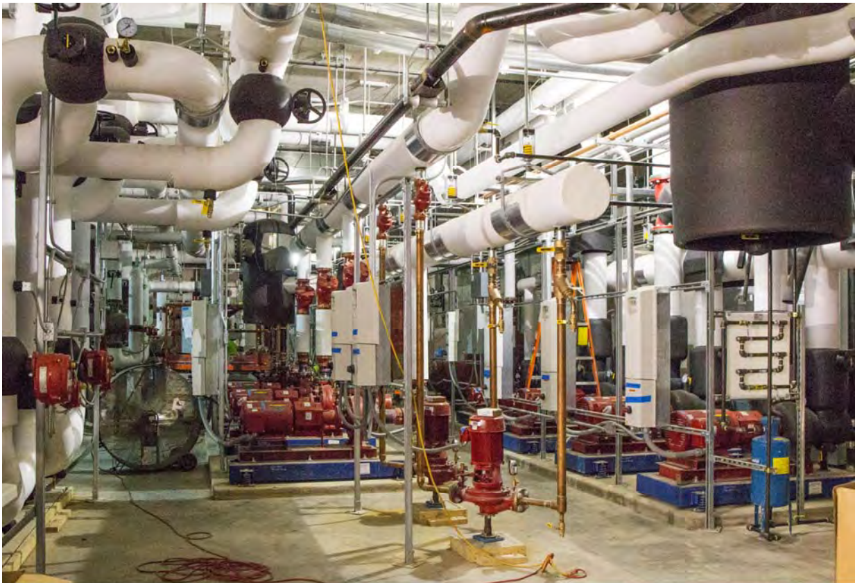
Hilton Cleveland Downtown, Cleveland, Ohio Contract Number: 140177 Photo 295 - HVAC System Piping Date: September 16, 2015
