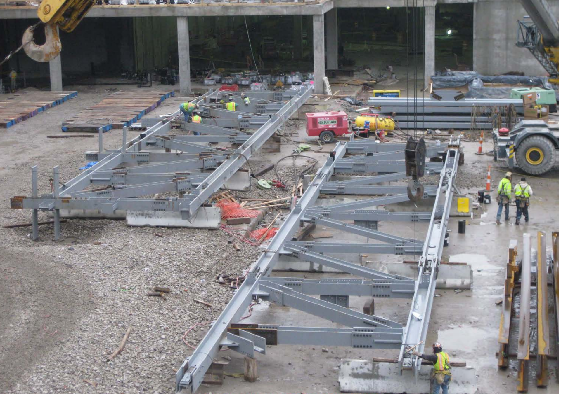
MEDICAL MART EAST TRUSS
