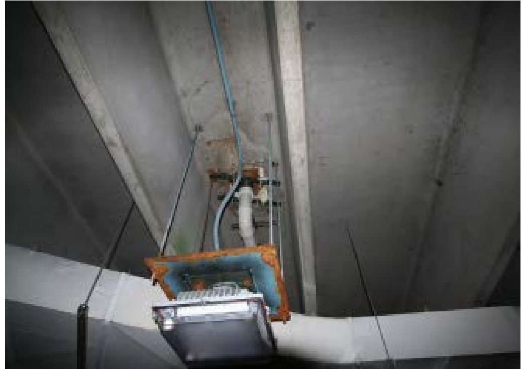
Typical leaking roof drain causing damage to structure
