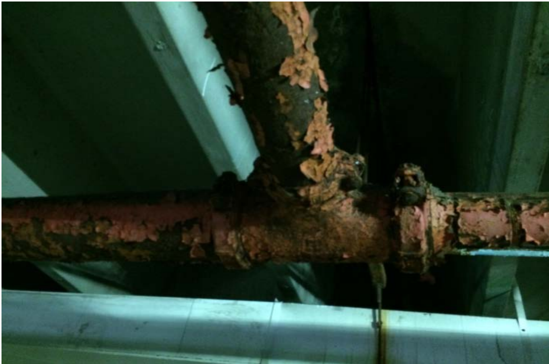
Extensive corrosion on FP mains, branch lines, fittings, and couplings
