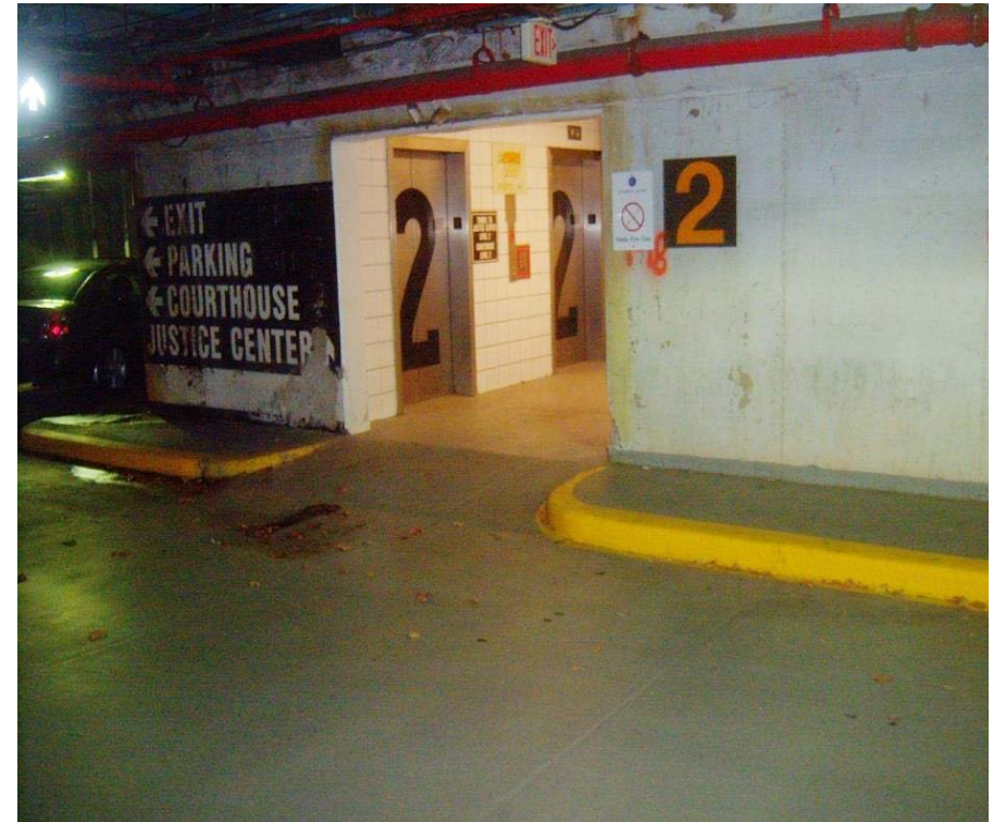
Typical non-compliant ramp
