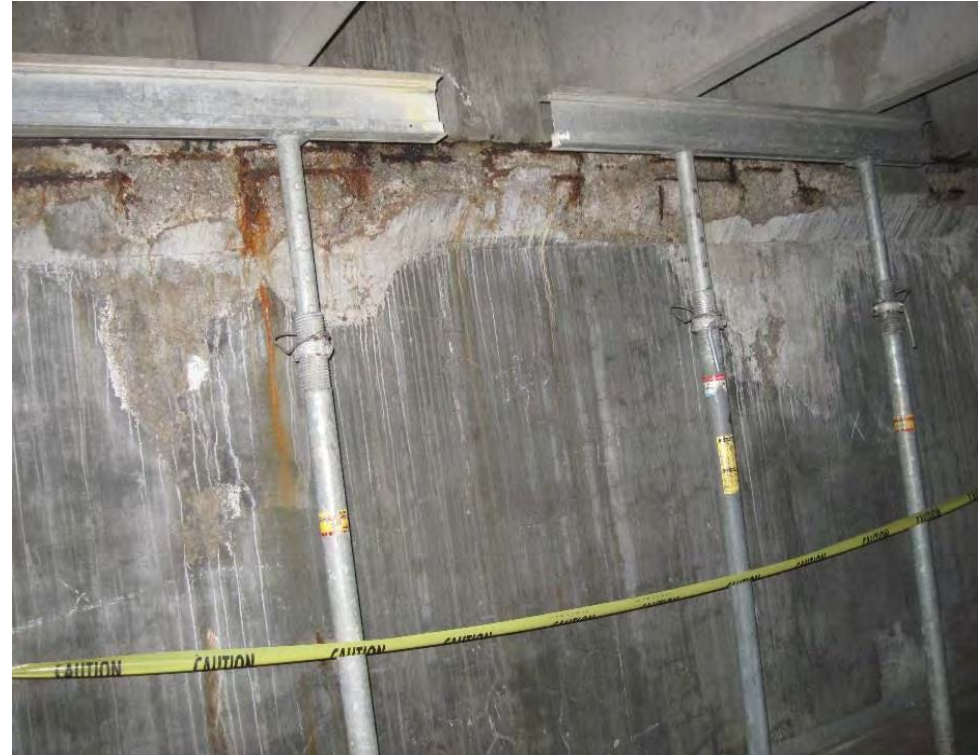
Concrete corbel with significant distress. Double tee beams required temporary shoring due to loss of bearing
