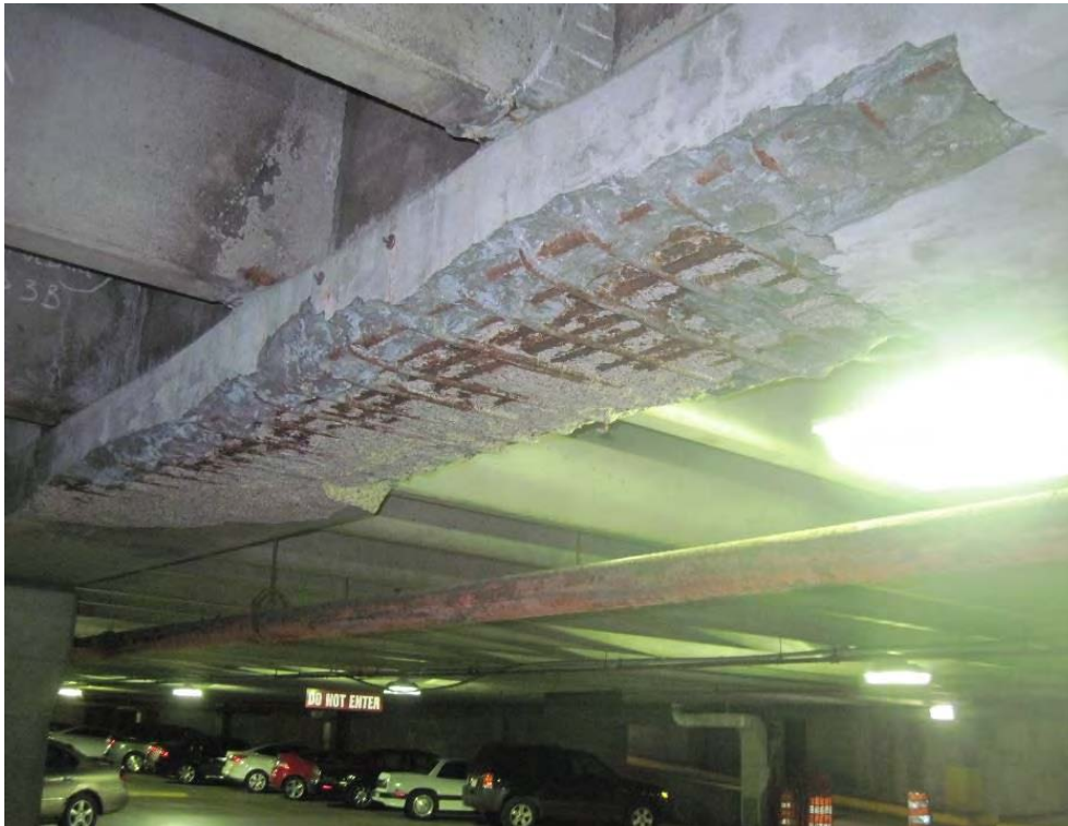
Girder with significant distress
