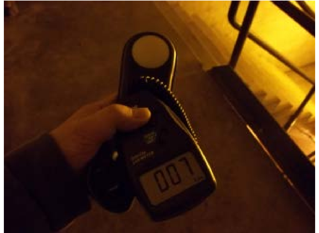
Inadequate lighting in stairwells
