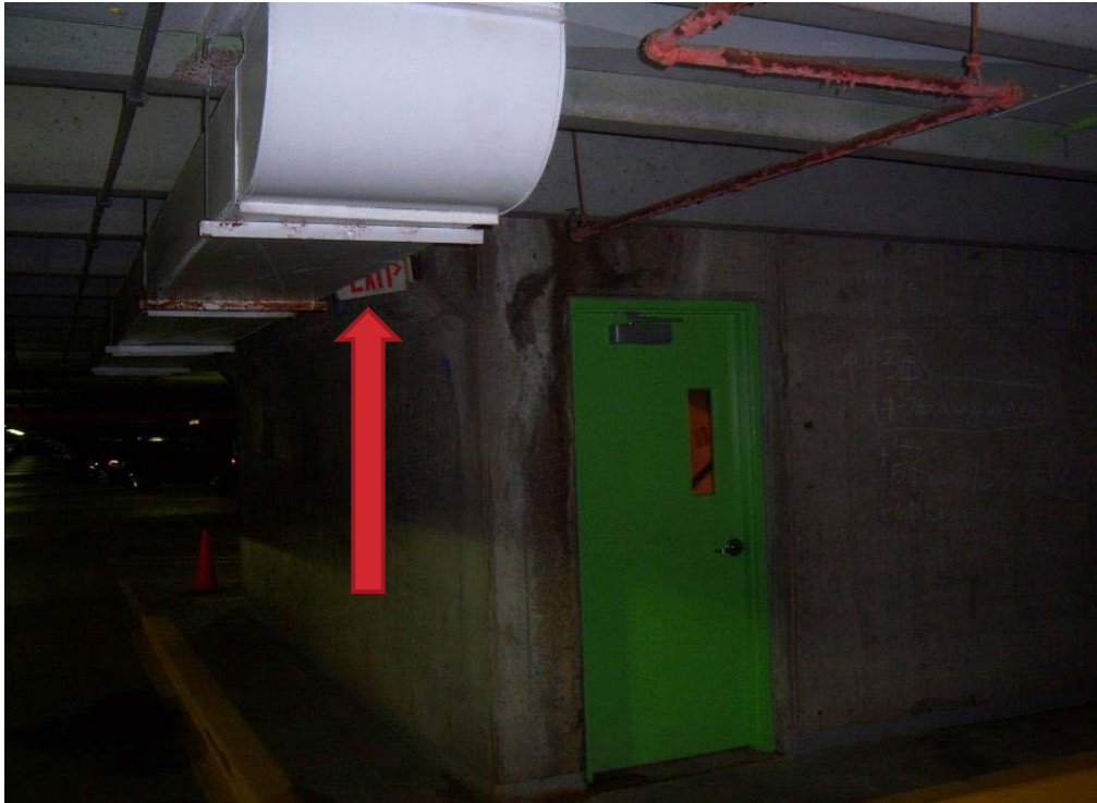
Exit path not visible, sign not illuminated and obstructed by existing ductwork
