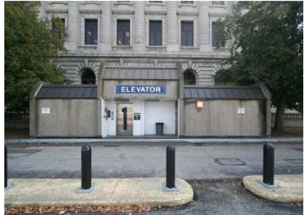
No roof drains or gutter to direct water away from sidewalk
