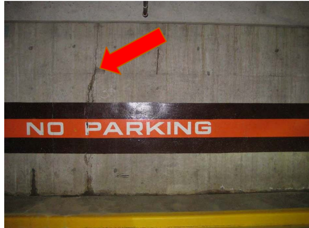
Concrete Wall crack with active water leakage
