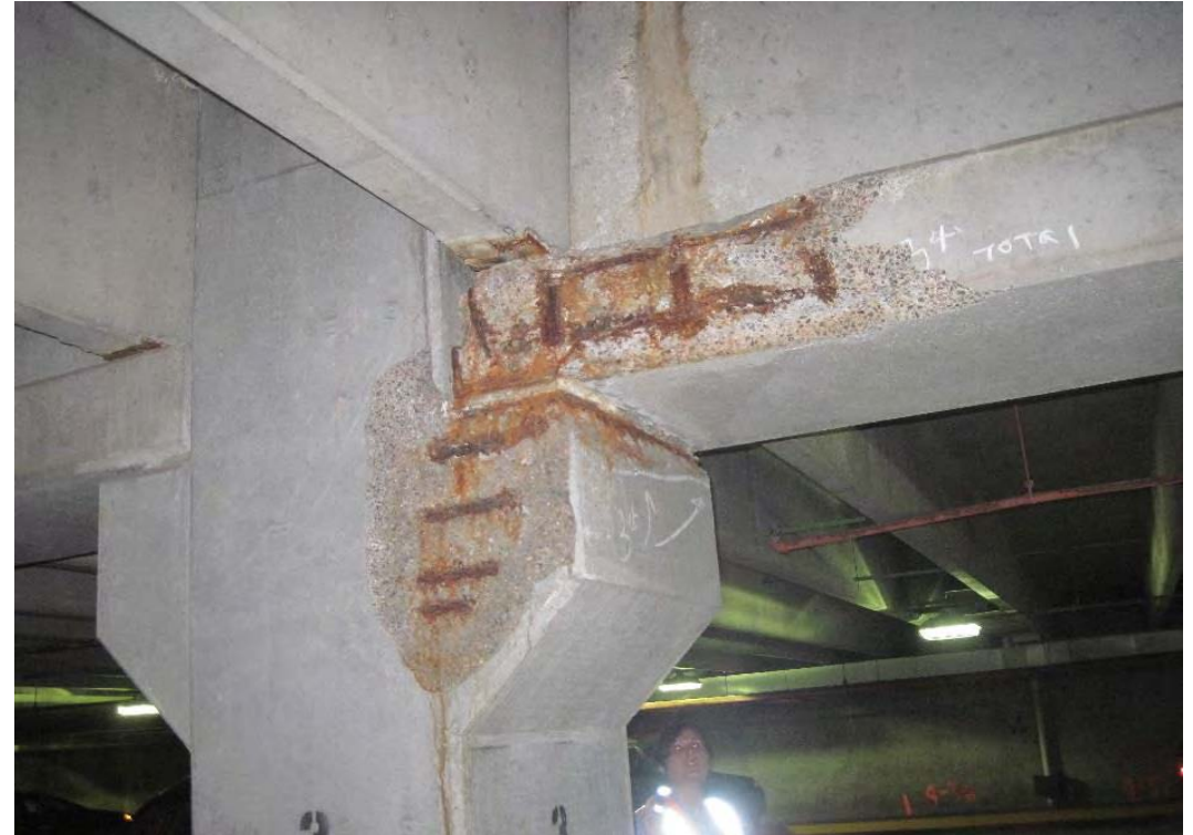
Typical distress at column corbel
