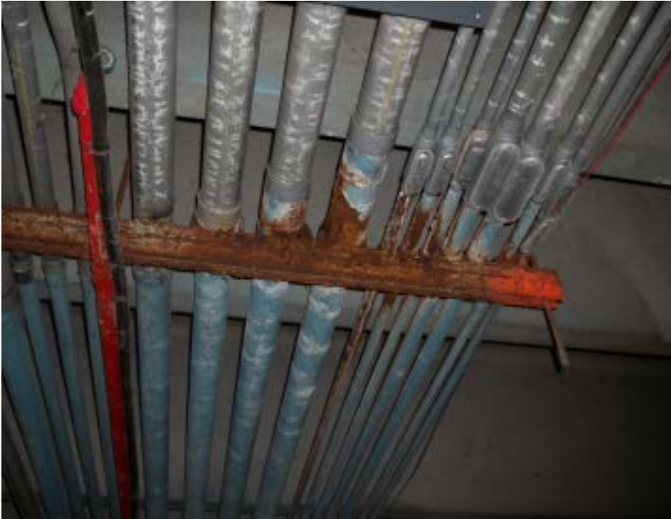
Corroded electrical conduits and hangar
