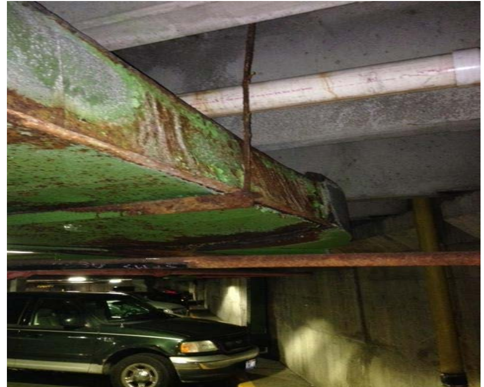
Deteriorated, collapsed duct main
