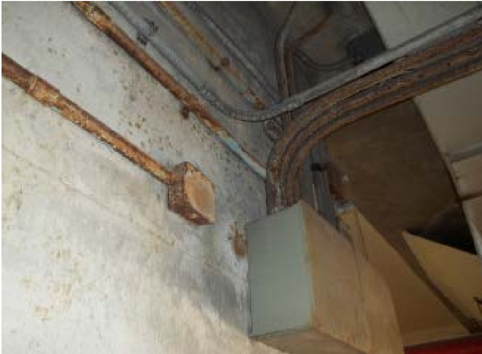
Corroded electrical conduits
