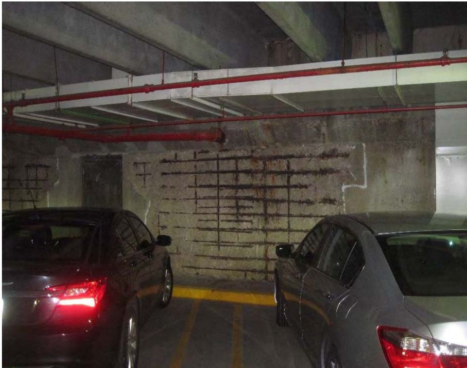
Concrete Wall distress showing delamination and exposed corroded reinforcing steel
