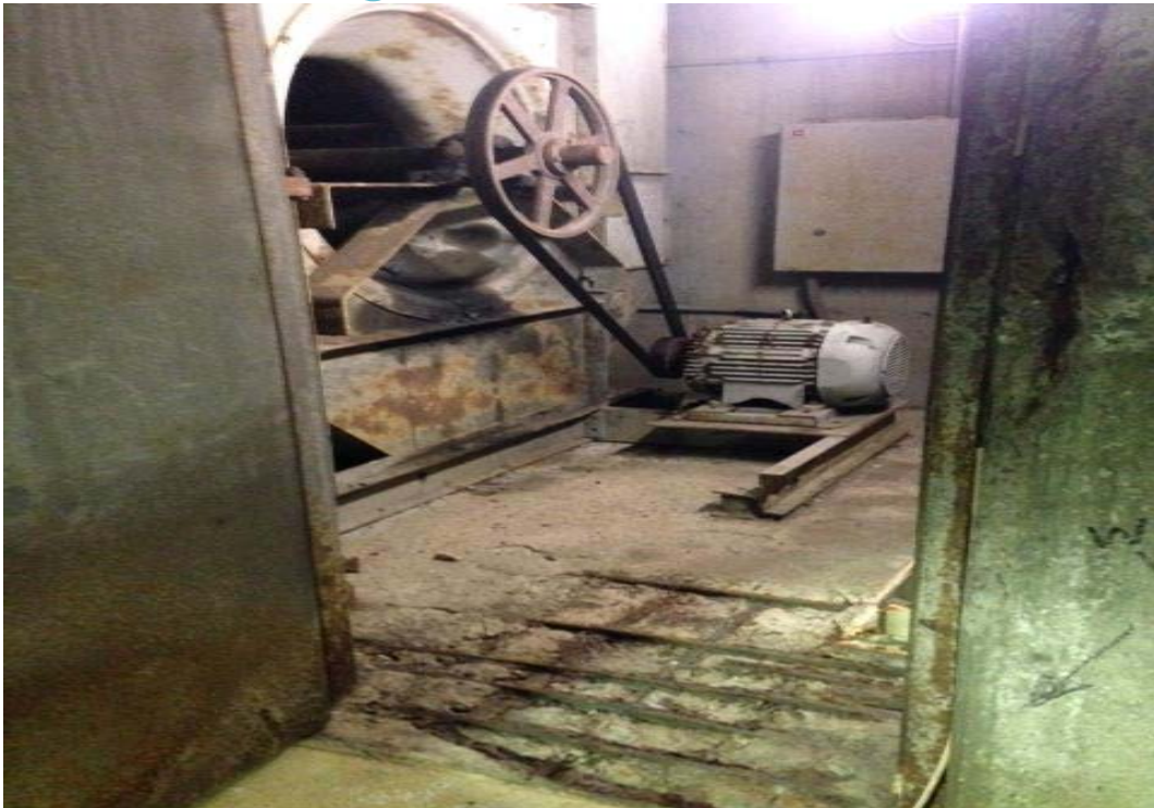
Exhaust fan and motor not performing properly. Need to be replaced.
