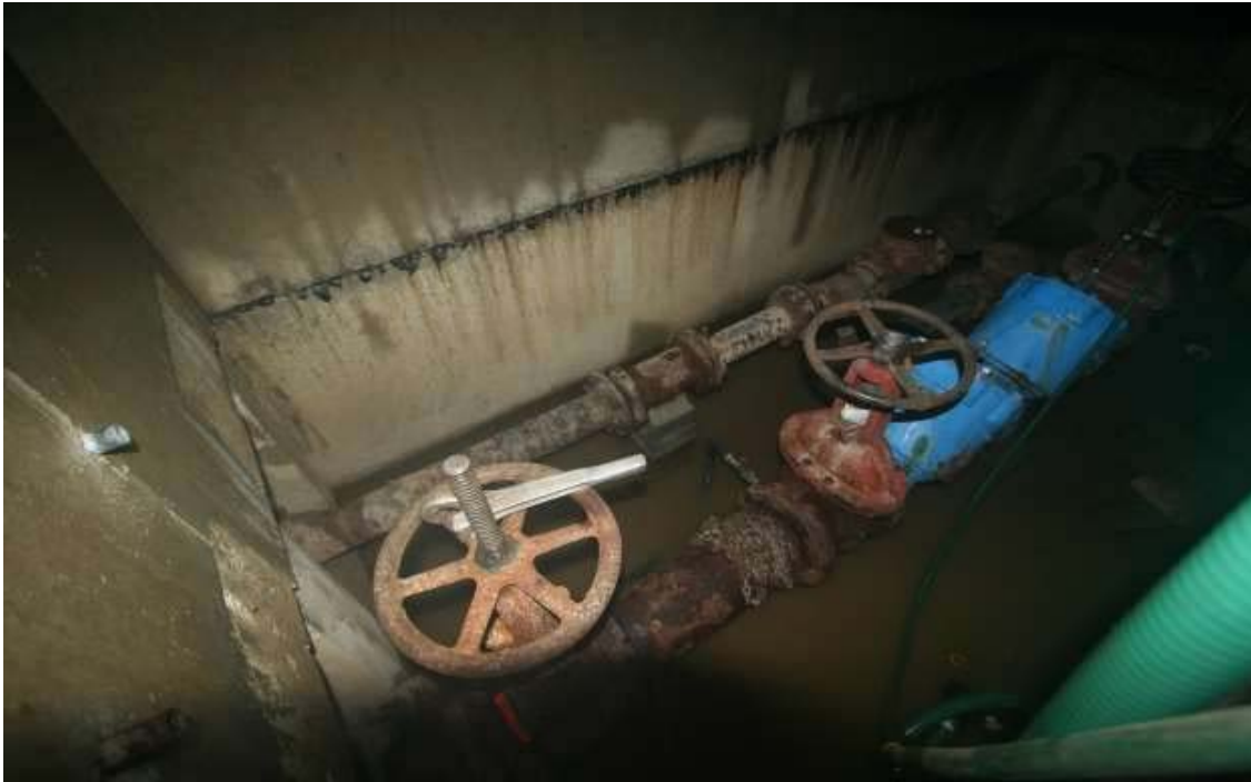
Extensive corrosion on FP mains, branch lines, fittings, and couplings
