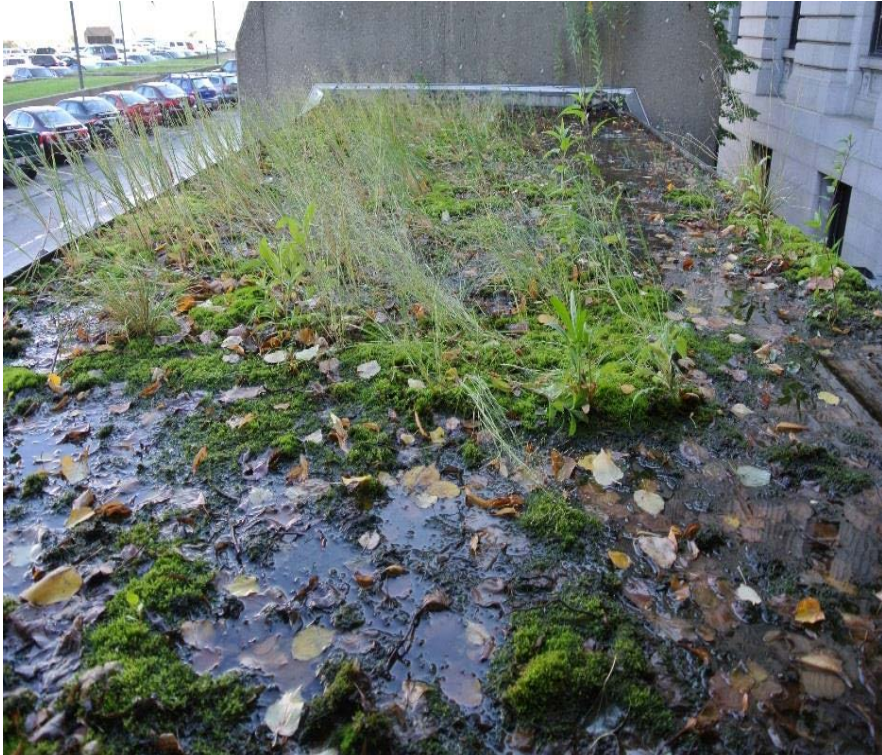
Ponding water and vegetation at roof penthouse
