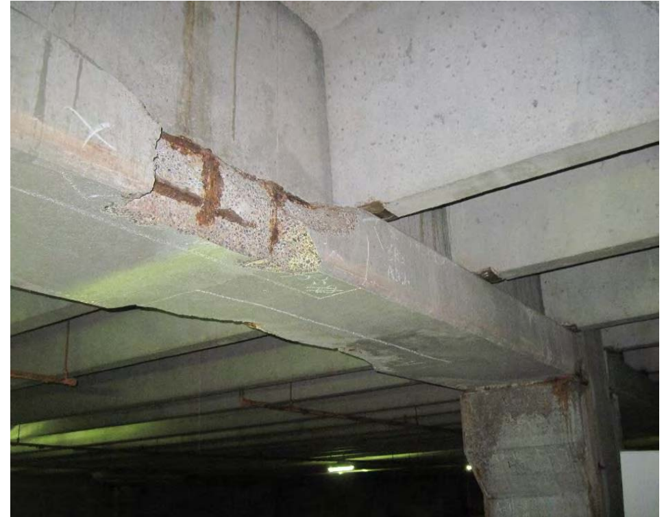
Typical distress at girder flange
