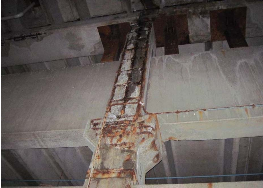
Concrete column with significant concrete loss and corroded reinforcing steel
