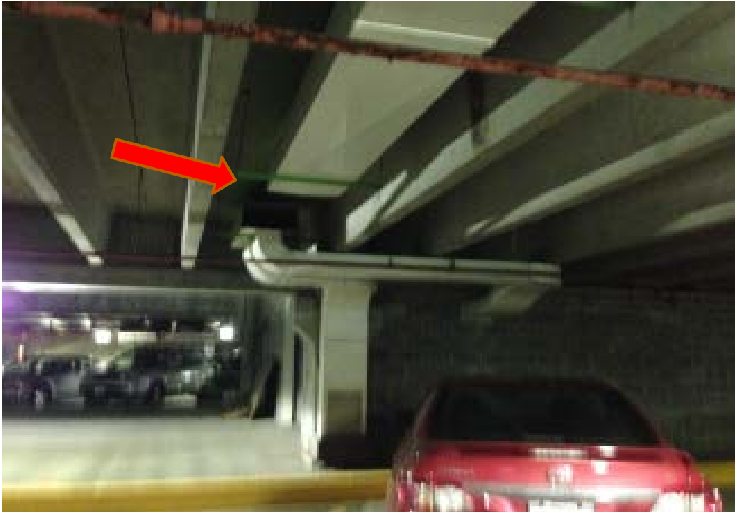
Exhaust duct branches missing
