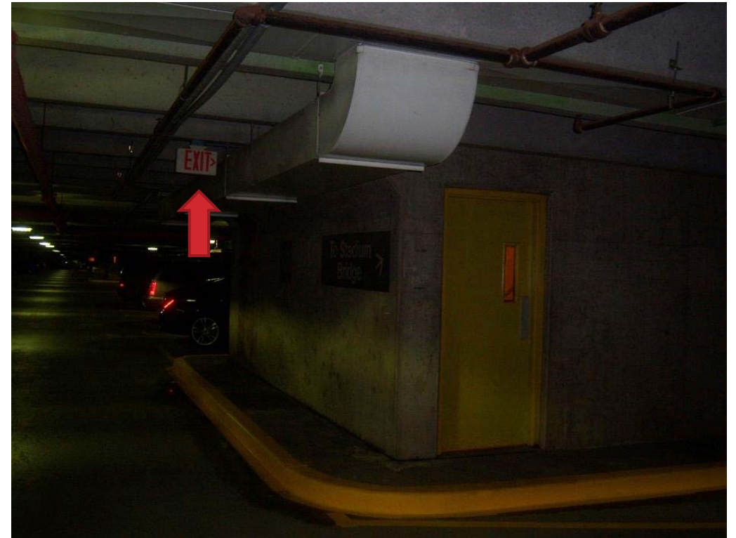
Exit sign not illuminated
