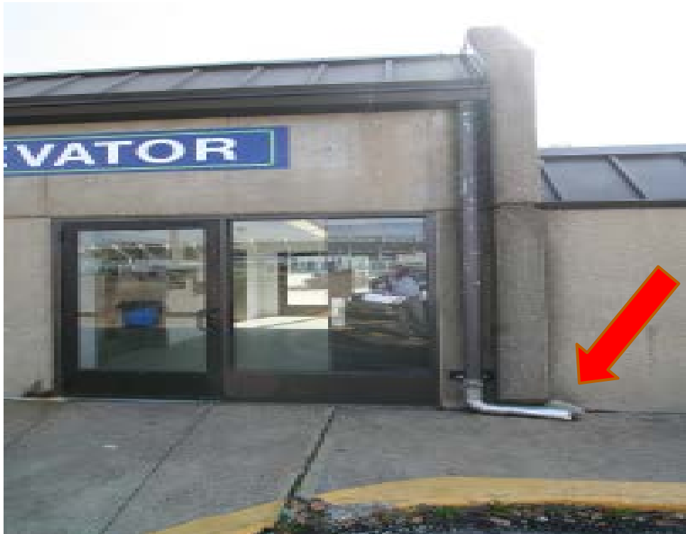
Gutter discharging to sidewalk
