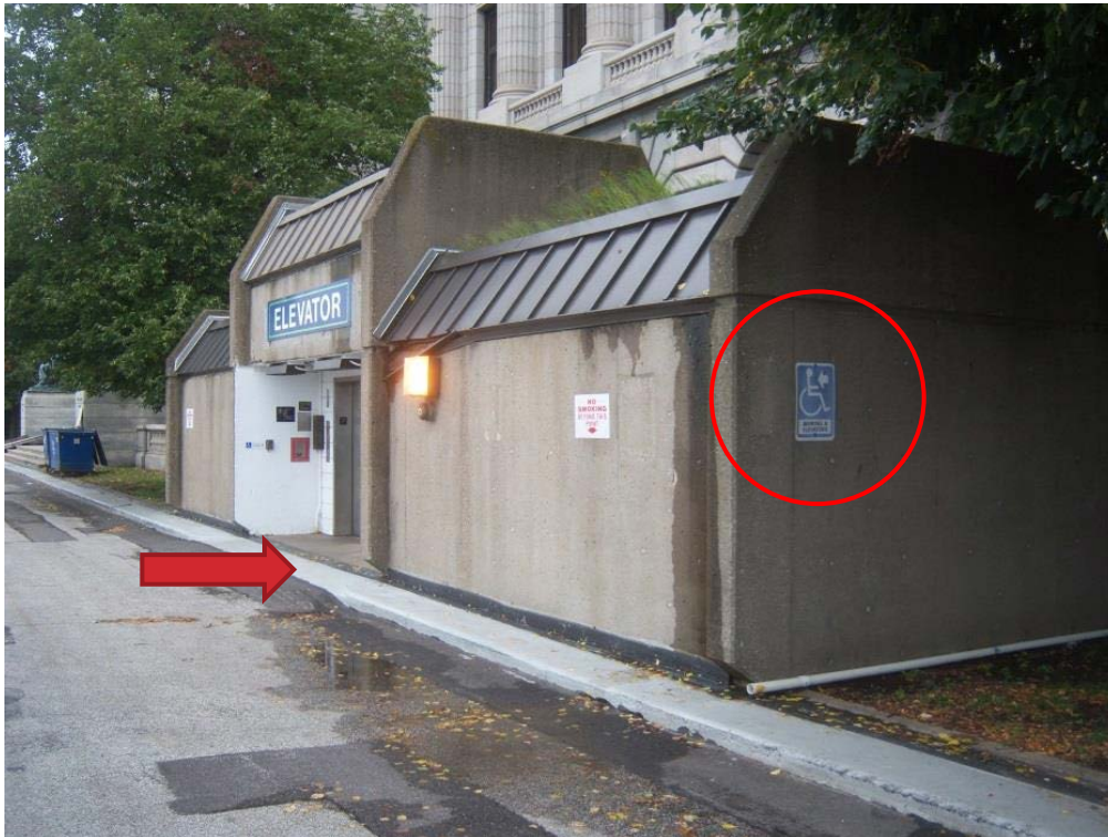
Poor visibility of accessible signage and call button; ramp to elevator is too steep and currently not enough room to install proper ramp
