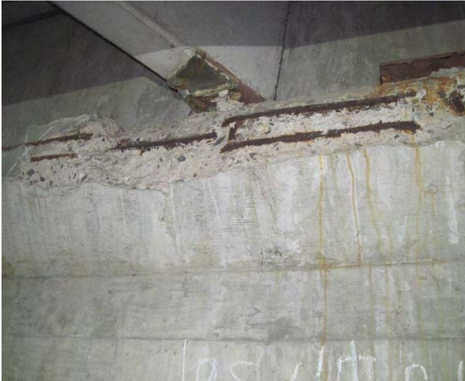
Typical concrete corbel distress with delaminated concrete and exposed reinforcing steel. Also, loss of bearing of double-tee stem
