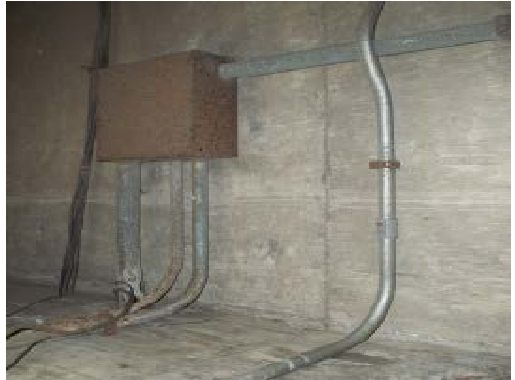
Typical outdated electrical equipment
