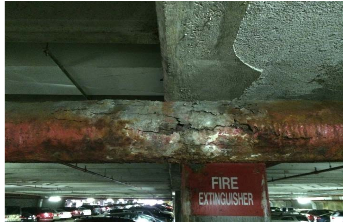
Typical extensive corrosion on mains for dry standpipe system.
