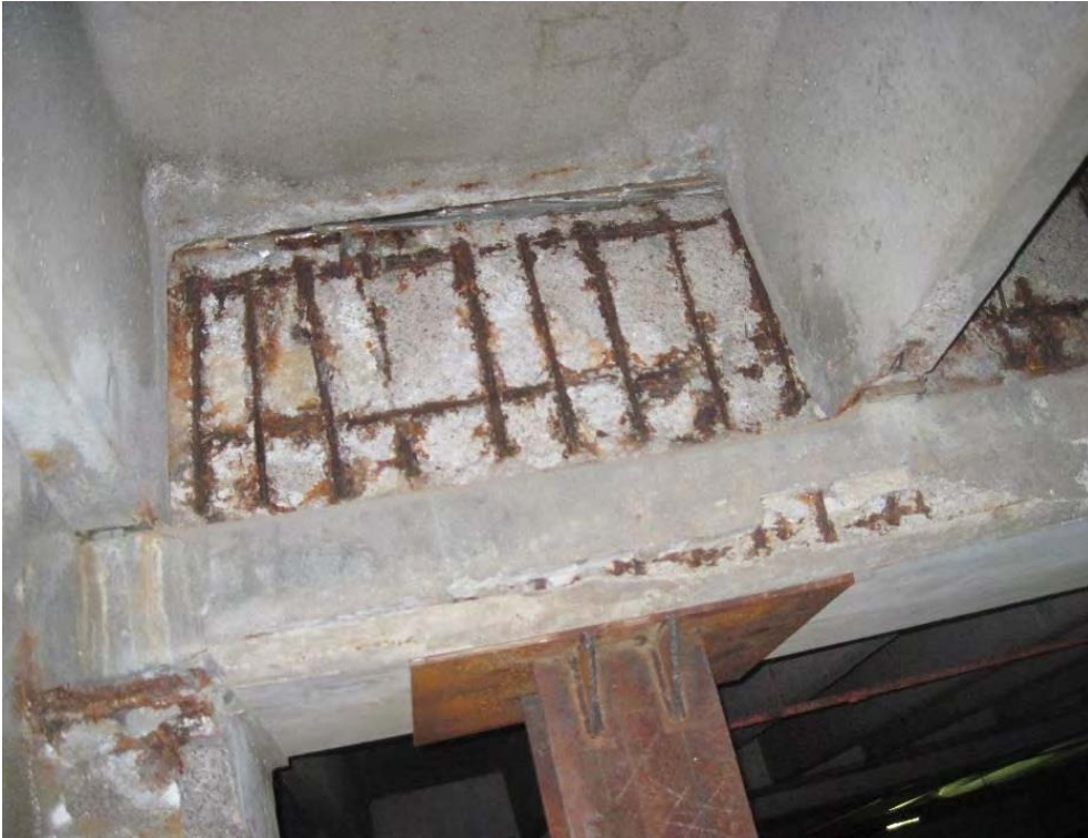
Girder required shoring due to web distress
