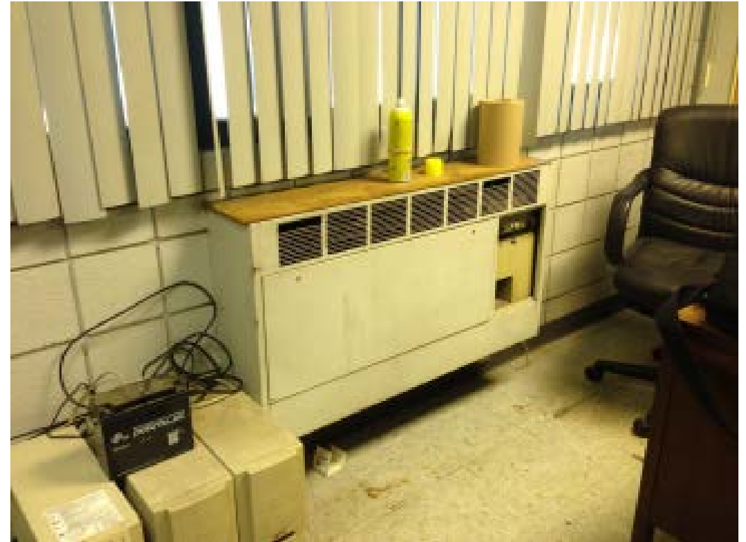
Electric cabinet heater units in need of replacement in office areas
