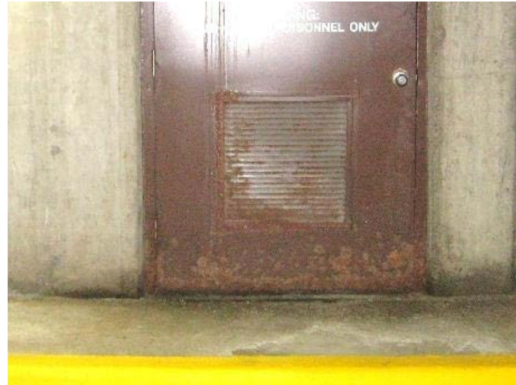
Typical corrosion at base of hinged door leaf, frame, and threshold
