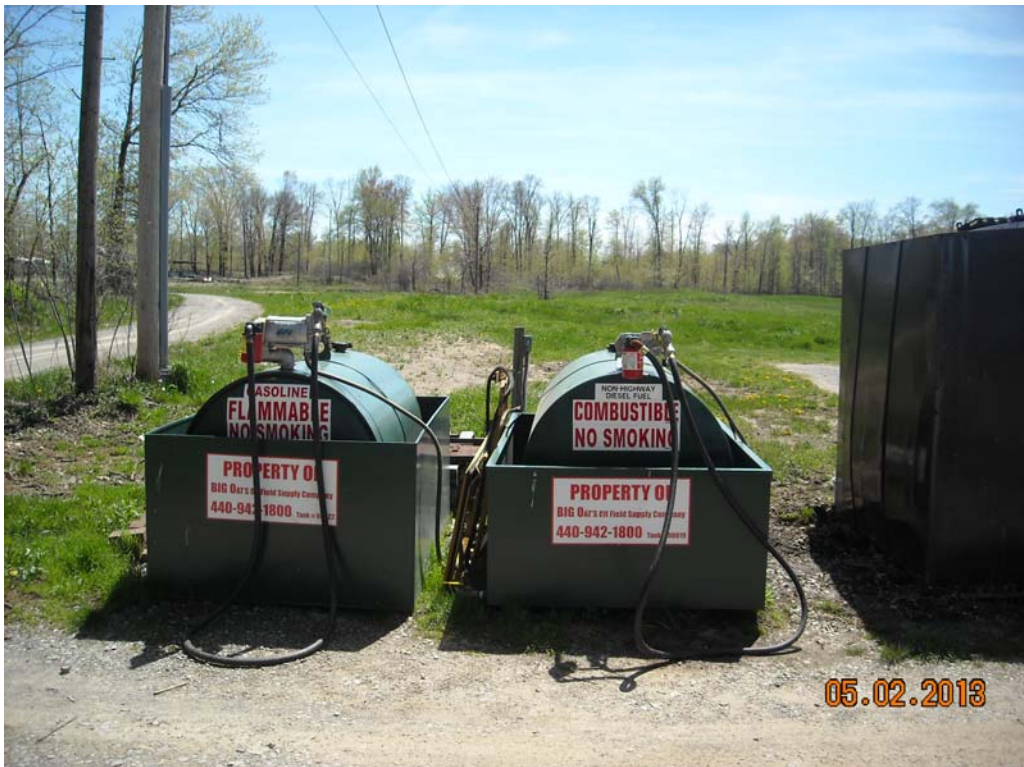
View of ASTs situated at the southeast corner of the subject property at Airport Greens Golf Course
