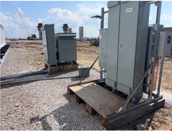
Temporary Power Gear
