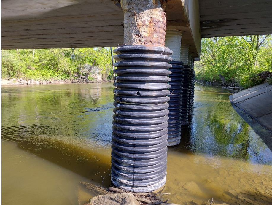
Photo 11 – Facing North - Bent 2, Pile 6. Missing top and bottom hose clamps on plastic pipe encasement.
