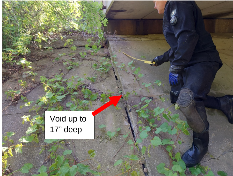
Photo 13 – Facing East – Void, cracking, and settlement of Forward Abutment slope protection (northeast corner).
