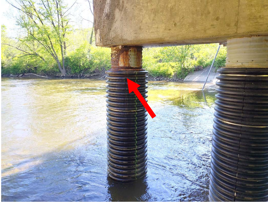
Photo 9 – Bent 1, Pile 1 – Missing hose clamp at top of plastic pipe encasement.
