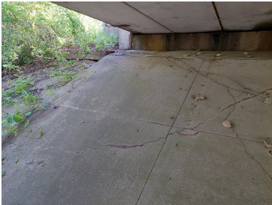
Photo 12 – Forward Abutment (east) slope protection – typical cracking.
