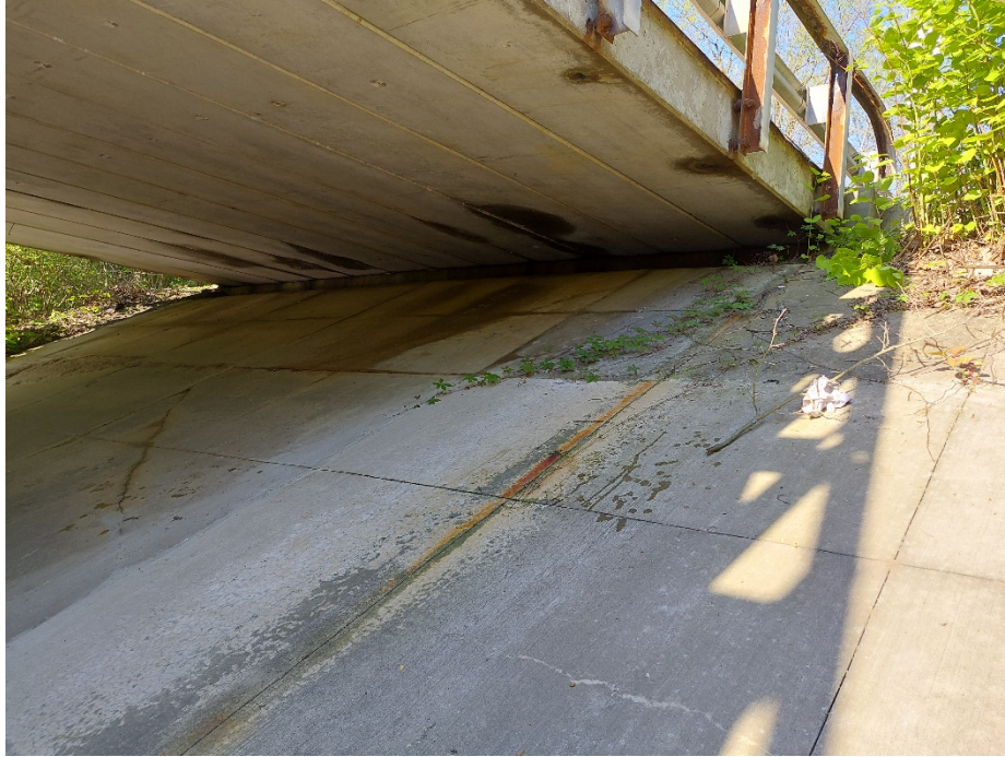
Photo 7 – Cracking and scaling of Rear Abutment (west) slope protection.
