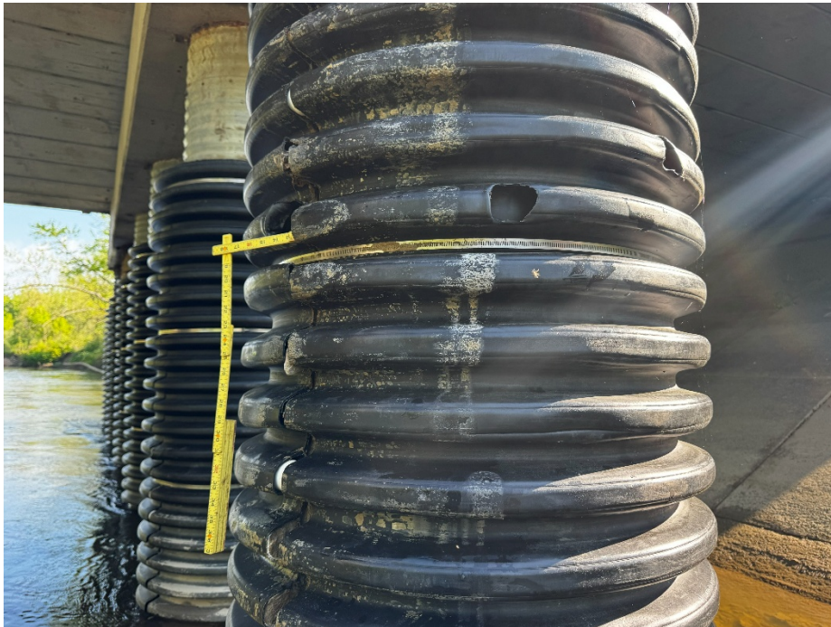
Photo 10 – Bent 2, Pile 6 – (3) 2" diameter holes in plastic pipe on upstream face of pile.
