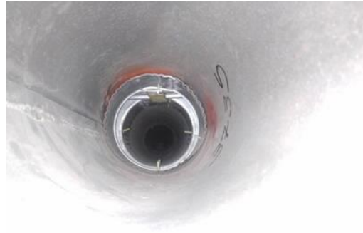
Picture of Damper in Open Position
