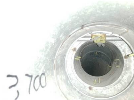
Picture of Damper in Closed Position
