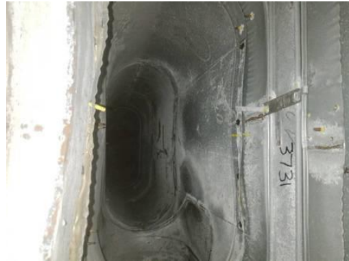
Picture of Damper in Closed Position
