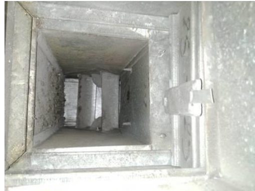
Picture of Damper in Closed Position
