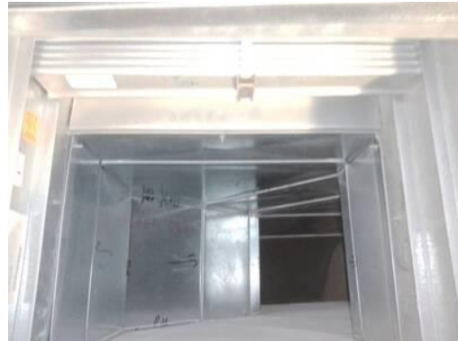
Picture of Damper in Closed Position
