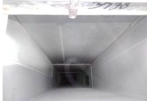
Picture of Damper in Closed Position
