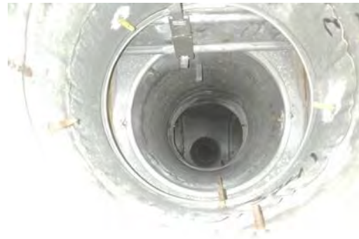
Picture of Damper in Open Position
