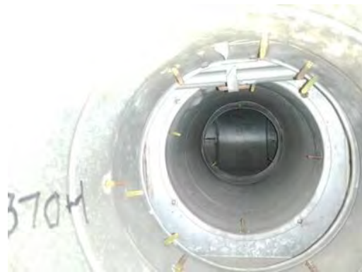
Picture of Damper in Closed Position
