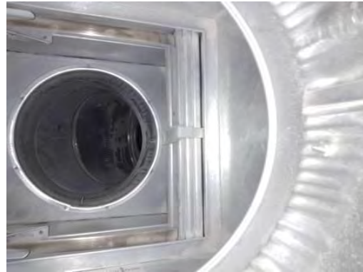
Picture of Damper in Closed Position
