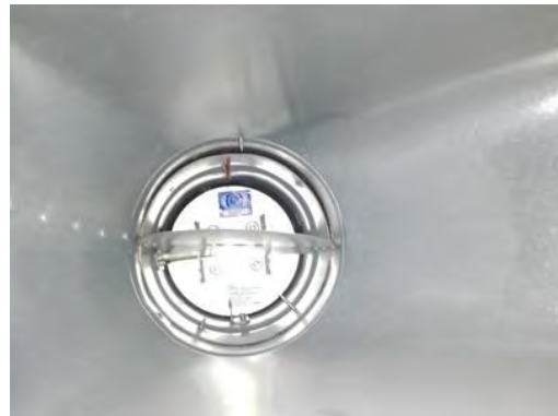
Picture of Damper I.D. Label
