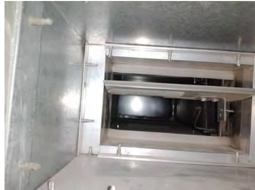
Picture of Damper in Closed Position
