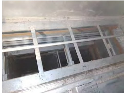
Picture of Damper in Closed Position
