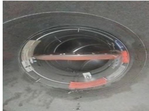
Picture of Damper in Closed Position
