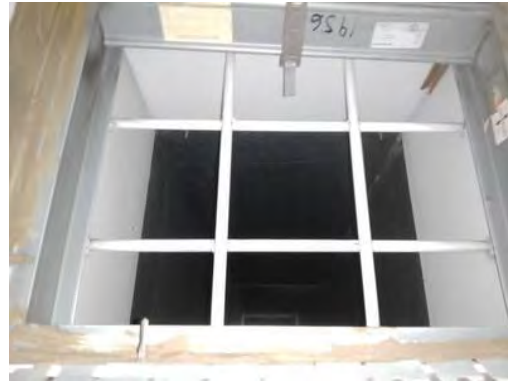
Picture of Damper in Closed Position
