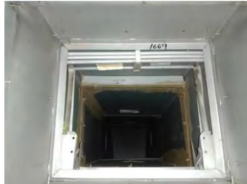
Picture of Damper in Closed Position
