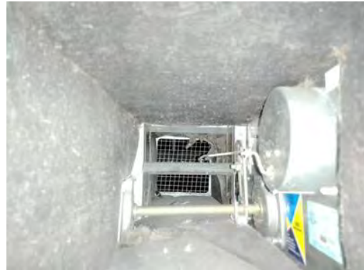
Picture of Damper in Closed Position
