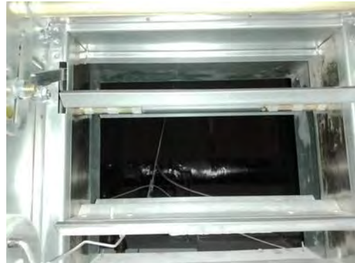
Picture of Damper in Closed Position
