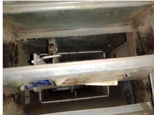
Picture of Damper in Closed Position
