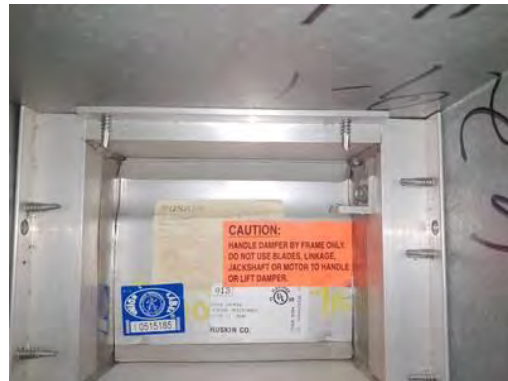
Picture of Damper I.D. Label
