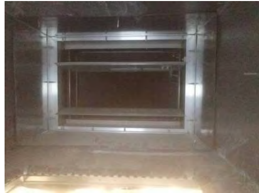
Picture of Damper in Closed Position
