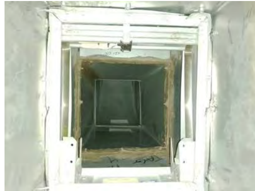
Picture of Damper in Closed Position
