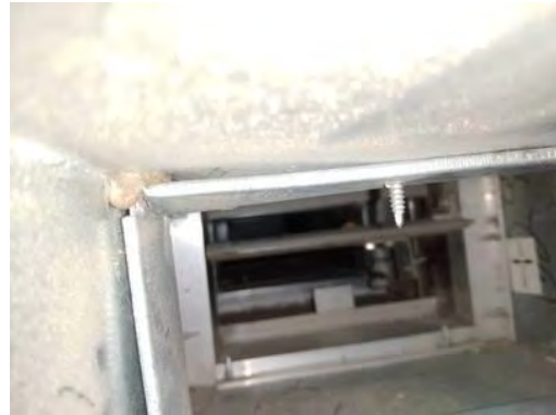
Picture of Damper in Closed Position
