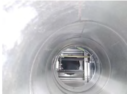
Picture of Damper in Closed Position
