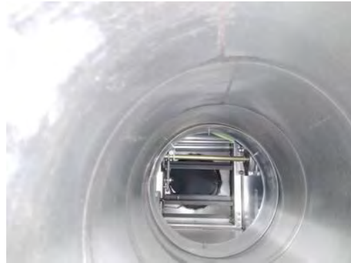
Picture of Damper in Closed Position
