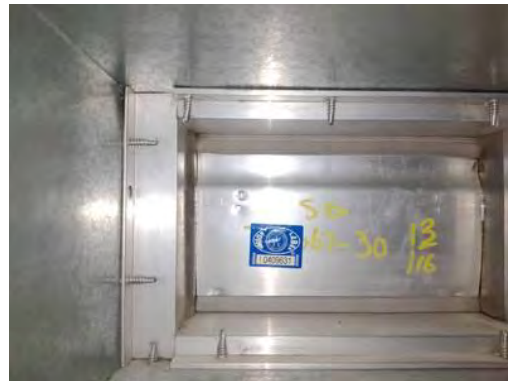
Picture of Damper I.D. Label
