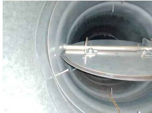
Picture of Damper in Closed Position
