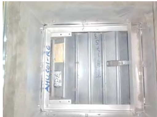
Picture of Damper I.D. Label
