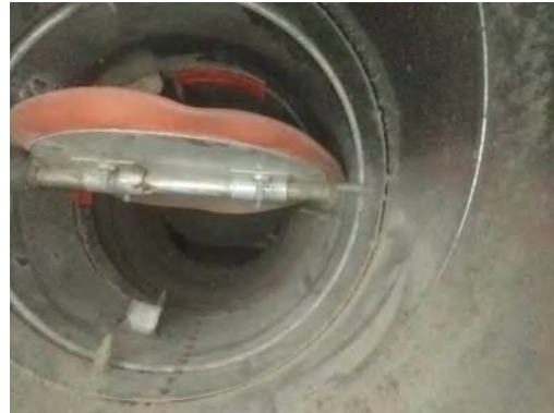
Picture of Damper in Closed Position
