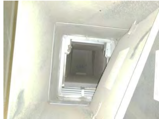
Picture of Damper in Closed Position
