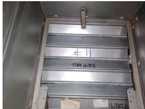
Picture of Damper I.D. Label
