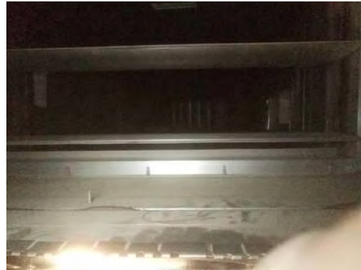
Picture of Damper in Closed Position
