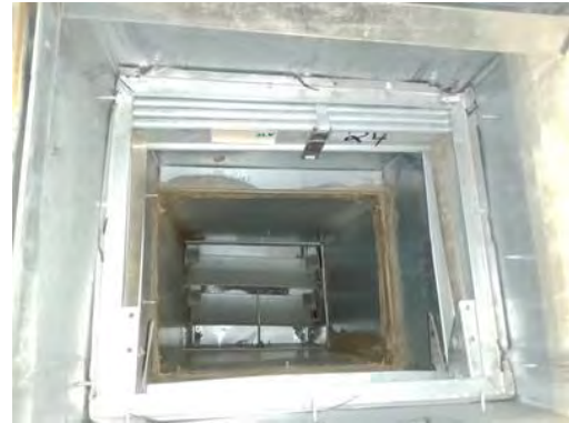
Picture of Damper in Closed Position
