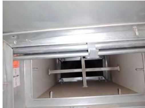
Picture of Damper in Closed Position
