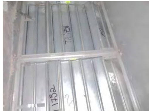
Picture of Damper I.D. Label
