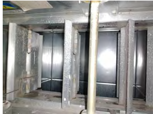
Picture of Damper in Closed Position
