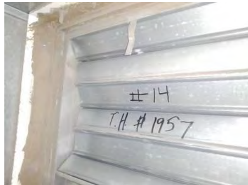
Picture of Damper I.D. Label
