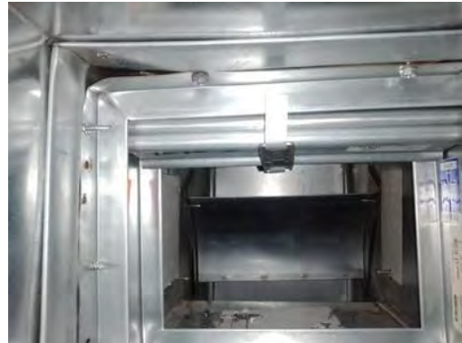
Picture of Damper in Closed Position
