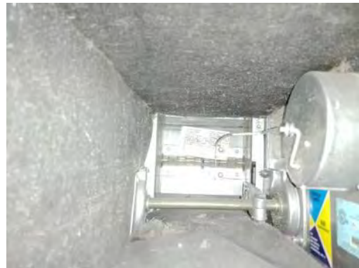
Picture of Damper I.D. Label
