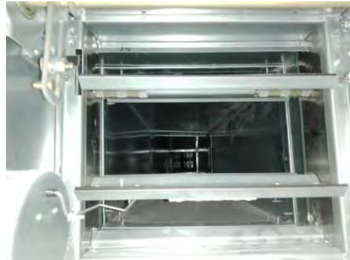
Picture of Damper in Closed Position
