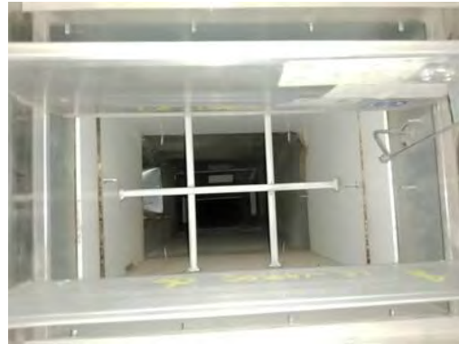
Picture of Damper in Closed Position
