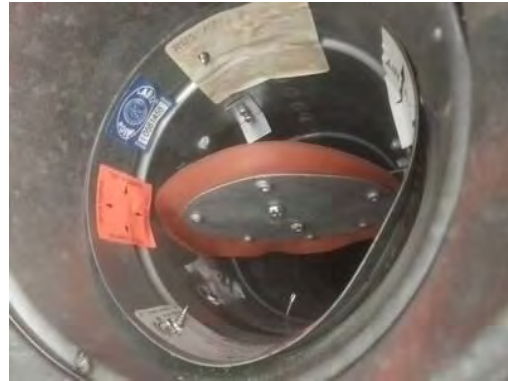
Picture of Damper in Closed Position
