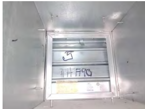
Picture of Damper I.D. Label
