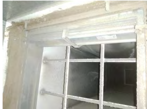
Picture of Damper in Closed Position
