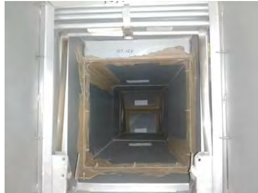
Picture of Damper in Closed Position
