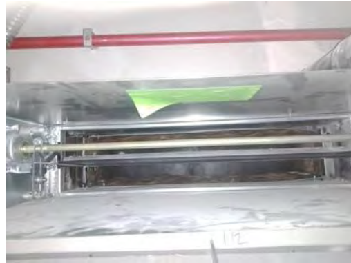
Picture of Damper in Closed Position
