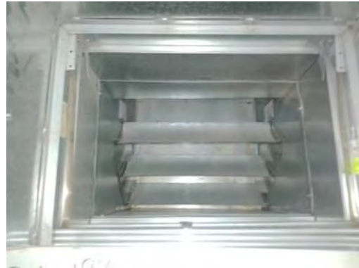
Picture of Damper in Closed Position
