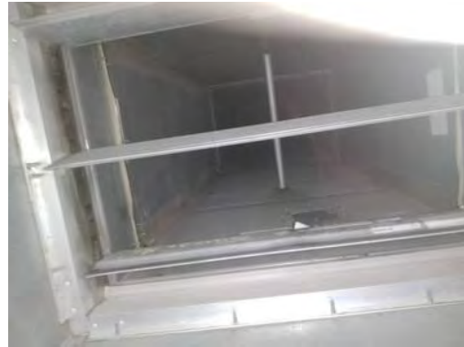
Picture of Damper in Closed Position
