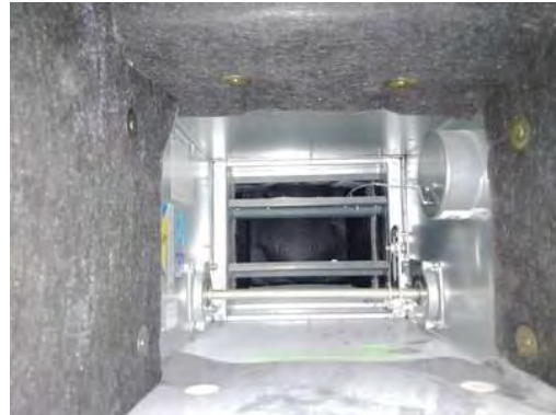
Picture of Damper in Closed Position
