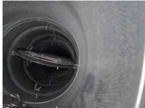
Picture of Damper in Closed Position
