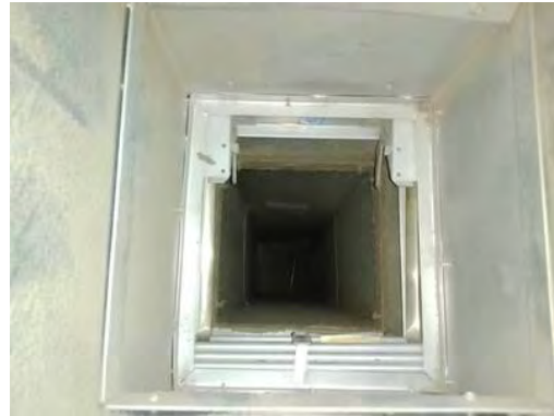
Picture of Damper in Closed Position
