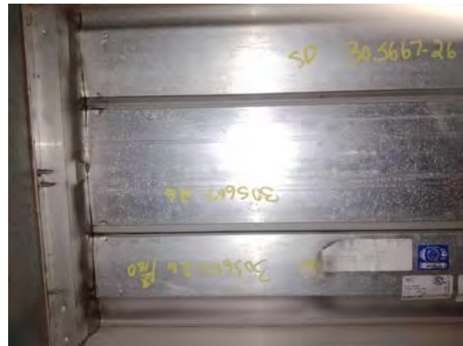
Picture of Damper I.D. Label
