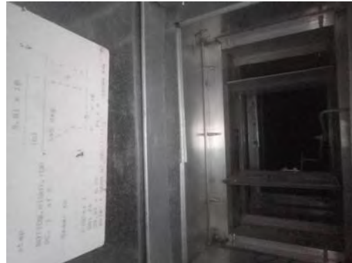
Picture of Damper in Closed Position
