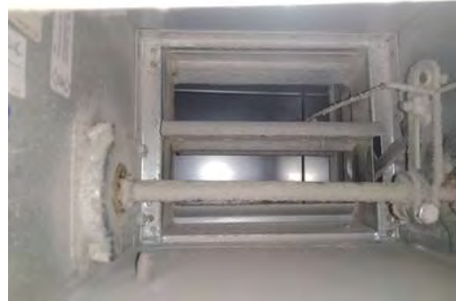
Picture of Damper in Closed Position
