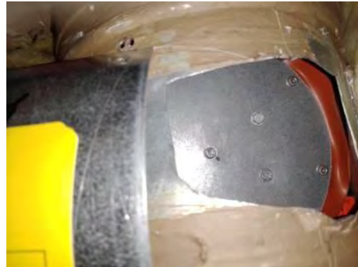
Picture of Damper in Closed Position
