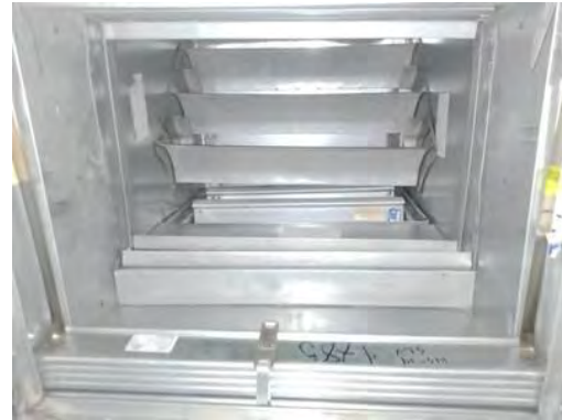
Picture of Damper in Closed Position
