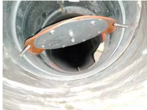
Picture of Damper in Closed Position
