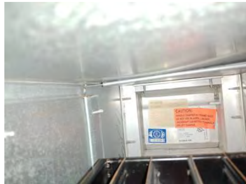
Picture of Damper I.D. Label
