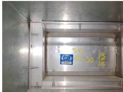
Picture of Damper I.D. Label
