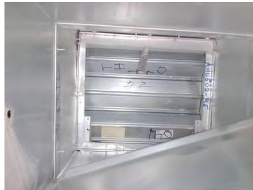
Picture of Damper I.D. Label
