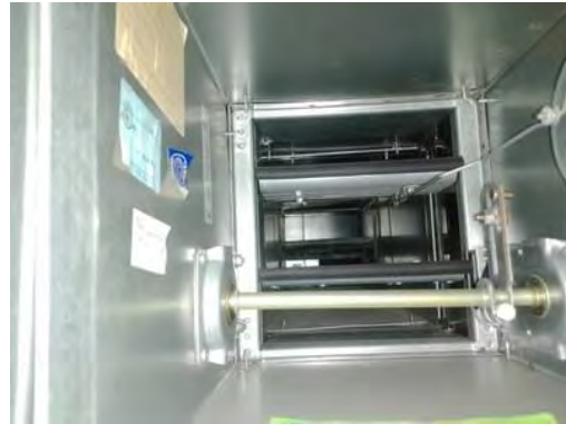
Picture of Damper in Closed Position
