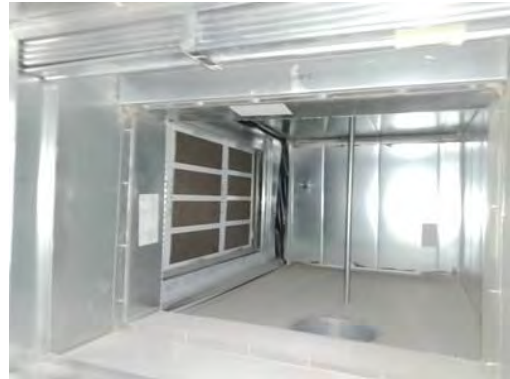
Picture of Damper in Closed Position
