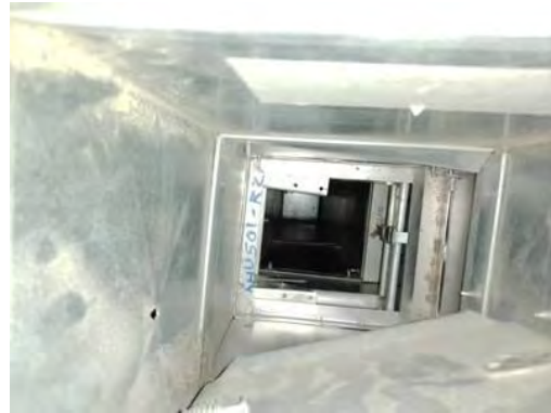
Picture of Damper in Closed Position
