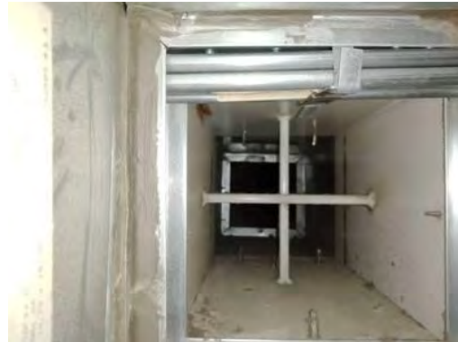
Picture of Damper in Closed Position
