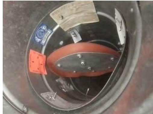
Picture of Damper in Closed Position
