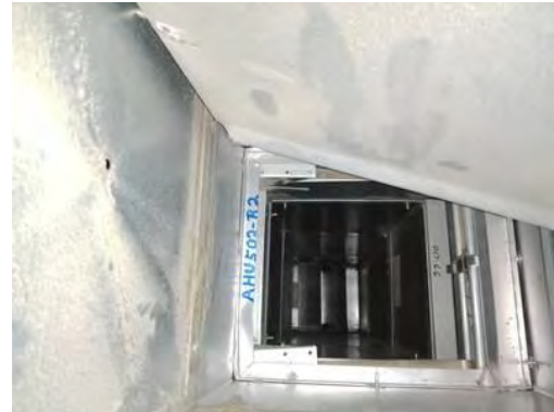
Picture of Damper in Closed Position
