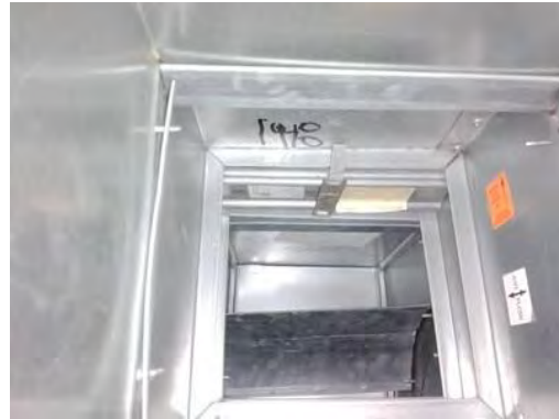
Picture of Damper in Closed Position
