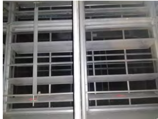
Picture of Damper in Closed Position
