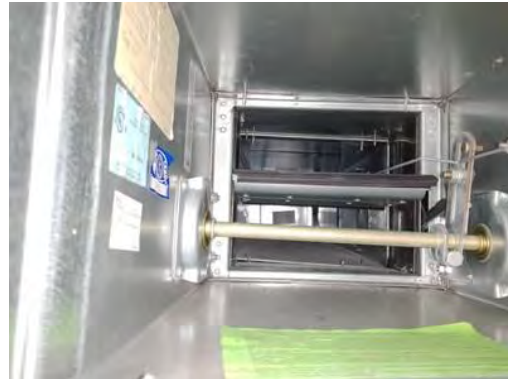
Picture of Damper in Closed Position
