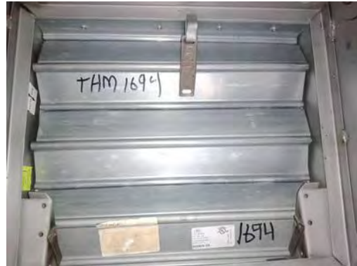
Picture of Damper I.D. Label
