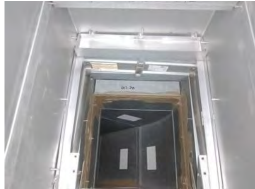
Picture of Damper in Closed Position
