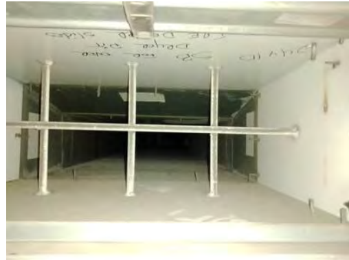
Picture of Damper in Closed Position
