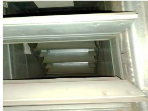
Picture of Damper in Closed Position
