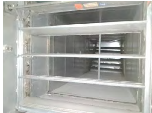
Picture of Damper in Closed Position
