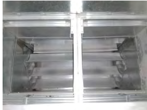
Picture of Damper in Closed Position
