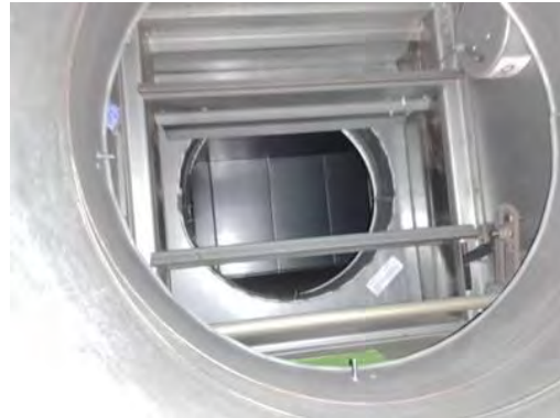
Picture of Damper in Closed Position
