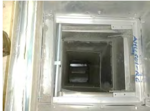
Picture of Damper in Closed Position
