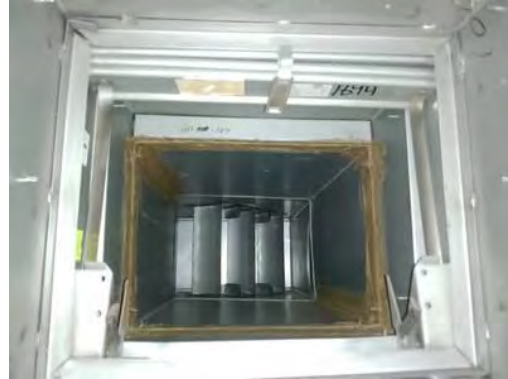
Picture of Damper in Closed Position
