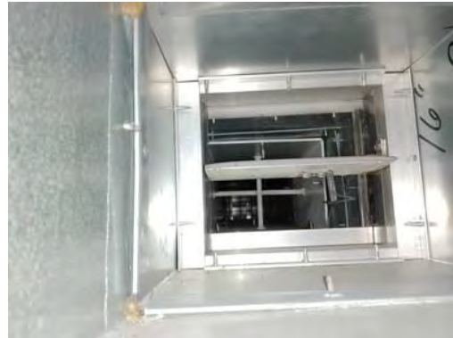
Picture of Damper in Closed Position
