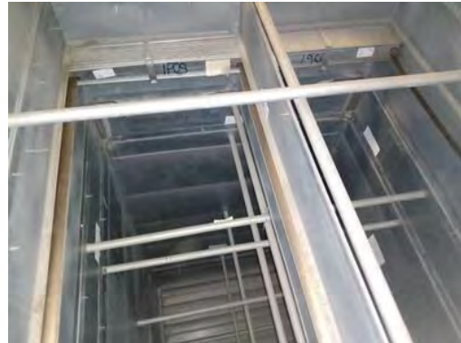
Picture of Damper in Closed Position
