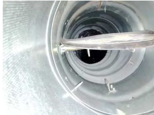
Picture of Damper in Closed Position
