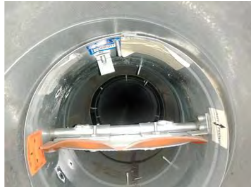
Picture of Damper in Closed Position
