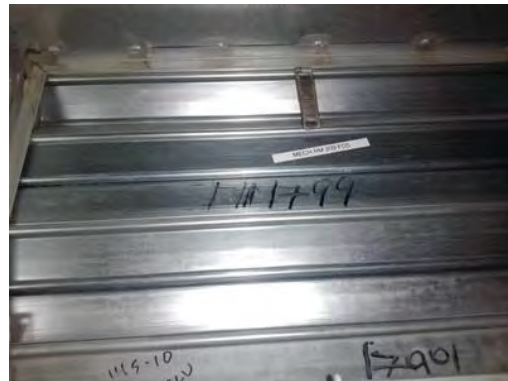
Picture of Damper I.D. Label
