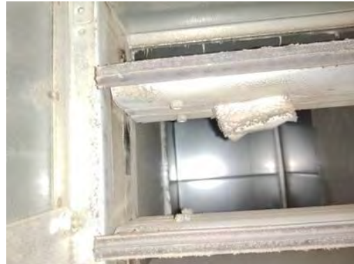
Picture of Damper in Closed Position
