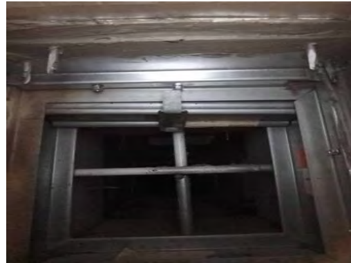
Picture of Damper in Closed Position
