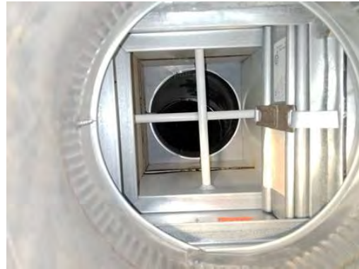
Picture of Damper in Closed Position
