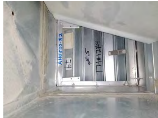
Picture of Damper I.D. Label
