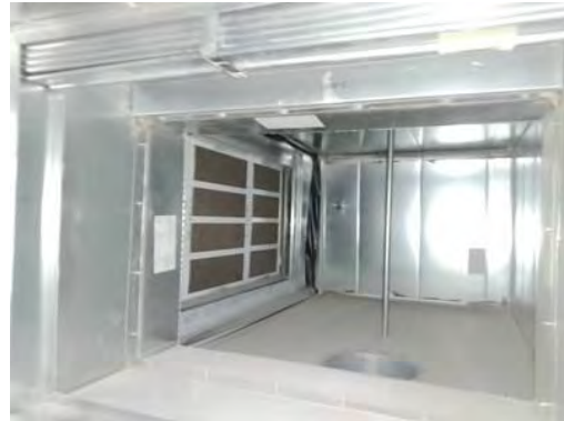
Picture of Damper in Closed Position
