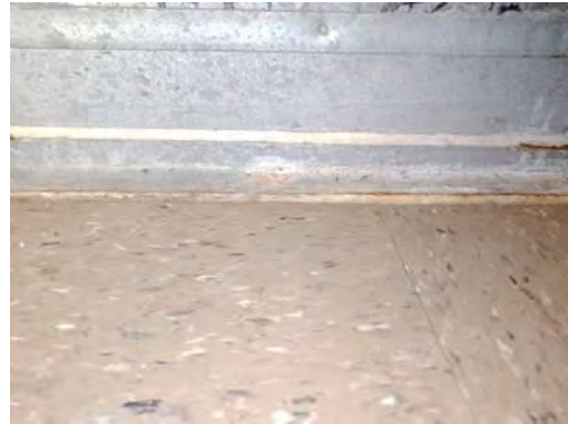
Picture of Damper in Closed Position
