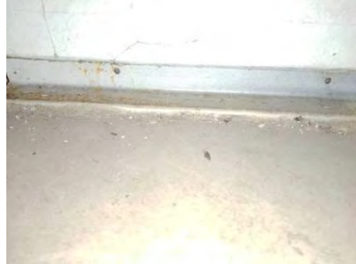
Interior Picture of Damper
