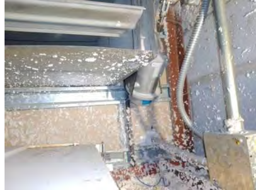
Interior Picture of Damper
