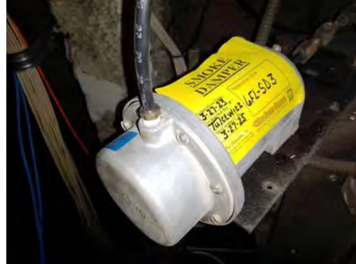
Interior Picture of Damper
