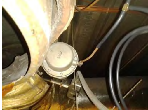
Interior Picture of Damper
