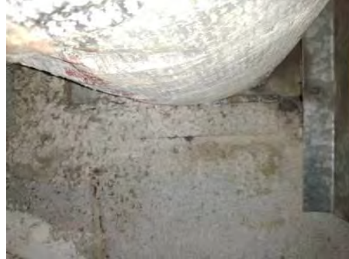
Interior Picture of Damper
