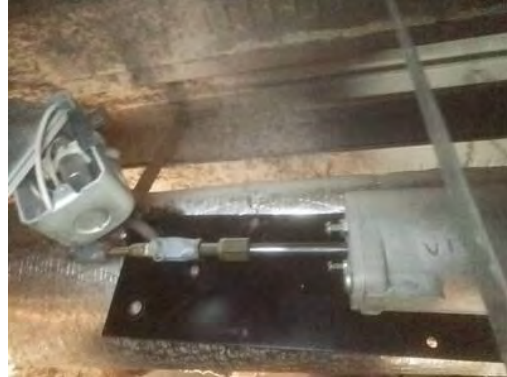
Interior Picture of Damper
