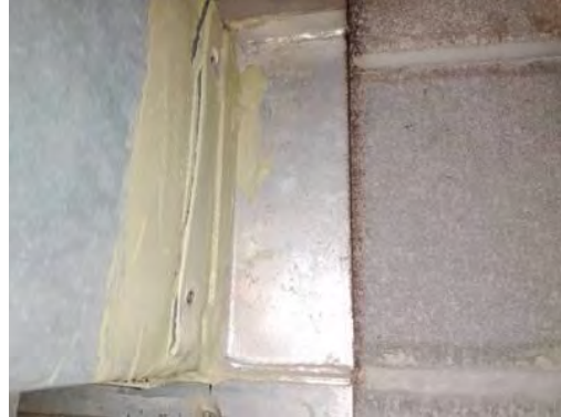
Interior Picture of Damper
