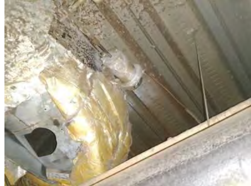
Interior Picture of Damper
