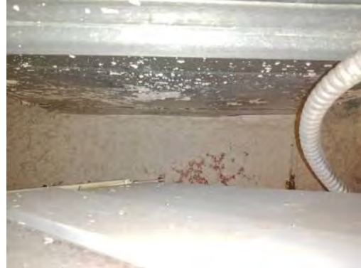
Interior Picture of Damper
