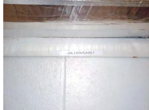
Interior Picture of Damper
