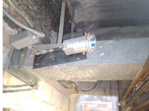
Interior Picture of Damper
