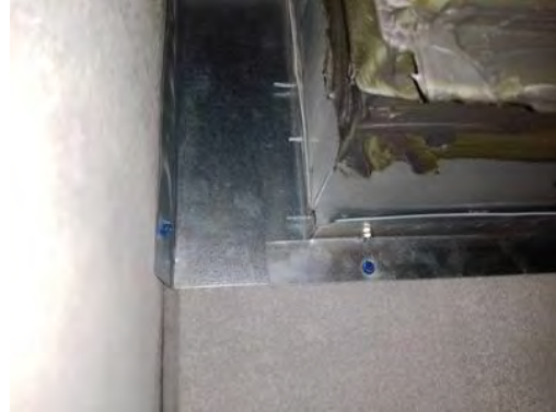
Interior Picture of Damper
