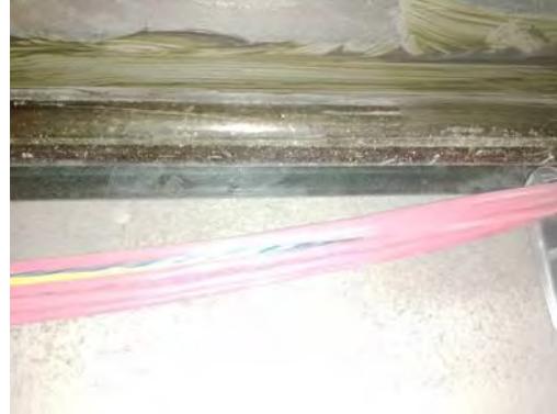
Interior Picture of Damper
