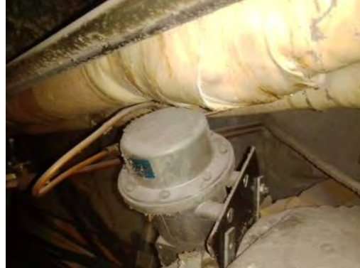
Interior Picture of Damper
