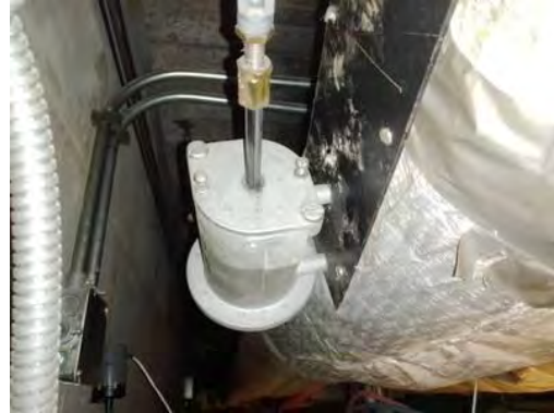
Interior Picture of Damper
