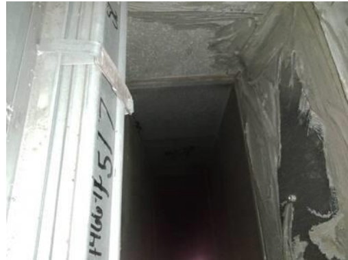
Picture of Damper in Closed Position
