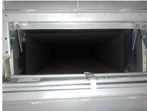
Picture of Damper in Closed Position
