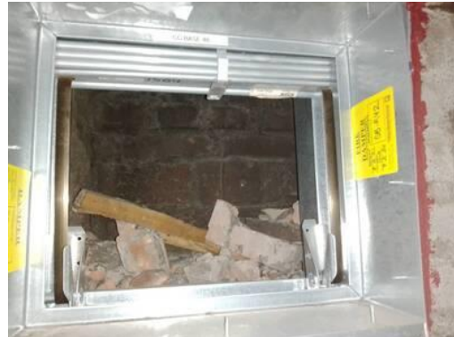
Picture of Damper in Closed Position
