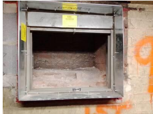
Picture of Damper in Closed Position
