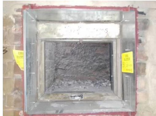
Picture of Damper in Closed Position
