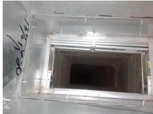
Picture of Damper in Closed Position
