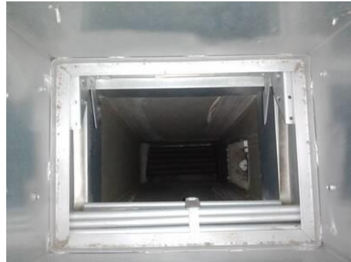
Picture of Damper in Closed Position
