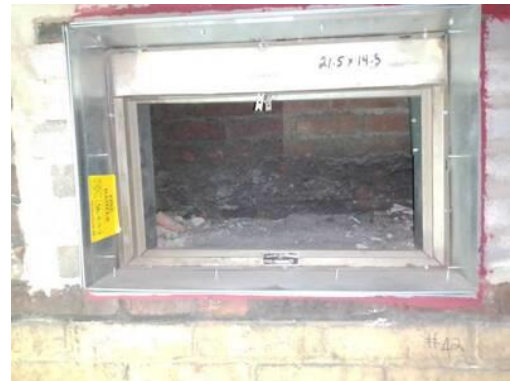
Picture of Damper in Closed Position
