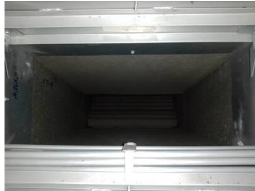
Picture of Damper in Closed Position
