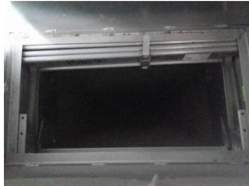
Picture of Damper in Closed Position
