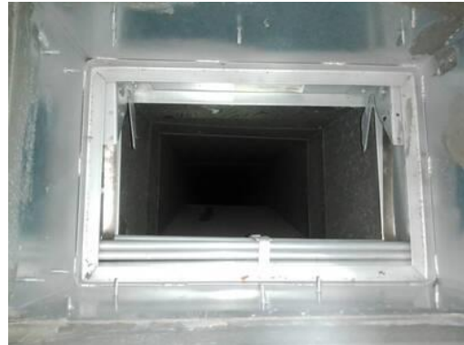
Picture of Damper in Closed Position
