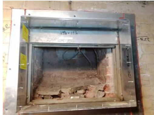
Picture of Damper in Closed Position
