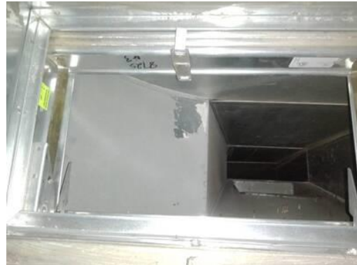
Picture of Damper in Closed Position
