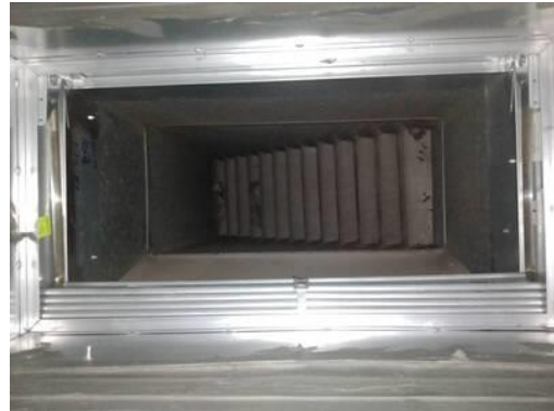
Picture of Damper in Closed Position
