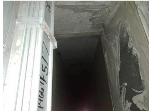
Picture of Damper in Closed Position
