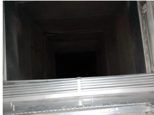
Picture of Damper in Closed Position
