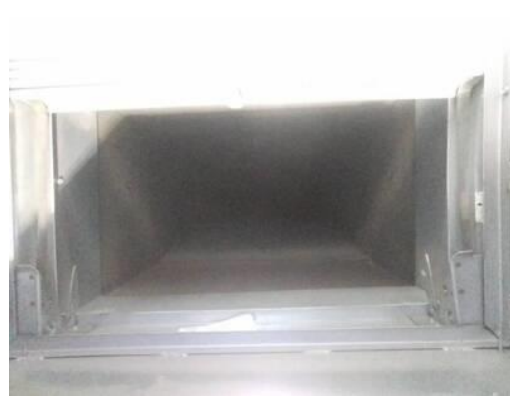
Picture of Damper in Closed Position
