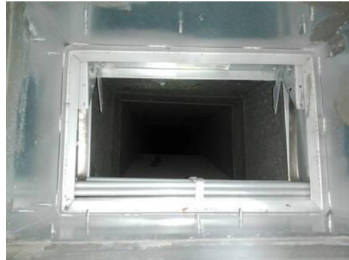
Picture of Damper in Closed Position
