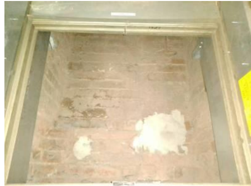
Picture of Damper in Closed Position
