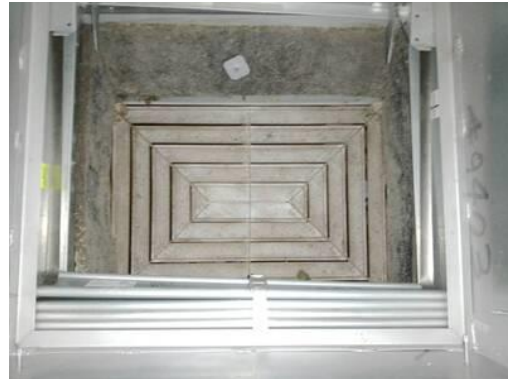
Picture of Damper in Closed Position
