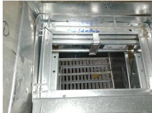
Picture of Damper in Closed Position
