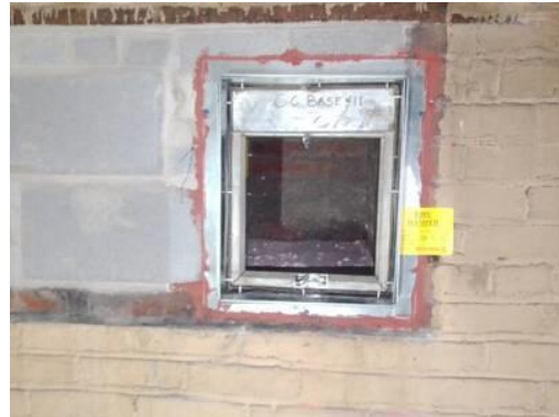
Picture of Damper in Closed Position
