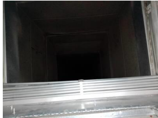
Picture of Damper in Closed Position
