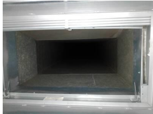
Picture of Damper in Closed Position
