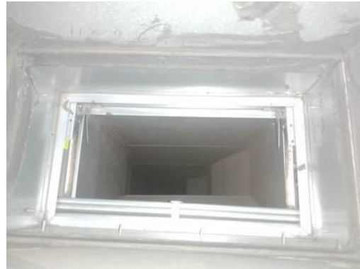
Picture of Damper in Closed Position
