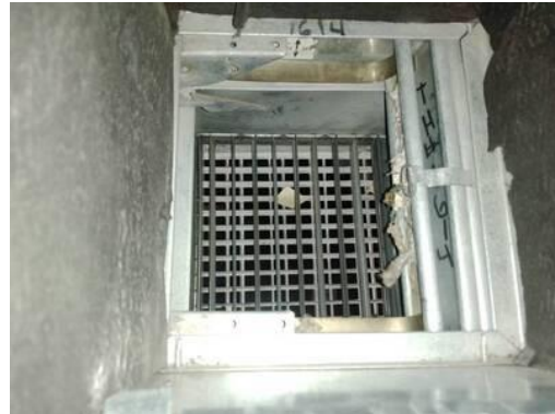
Picture of Damper in Closed Position
