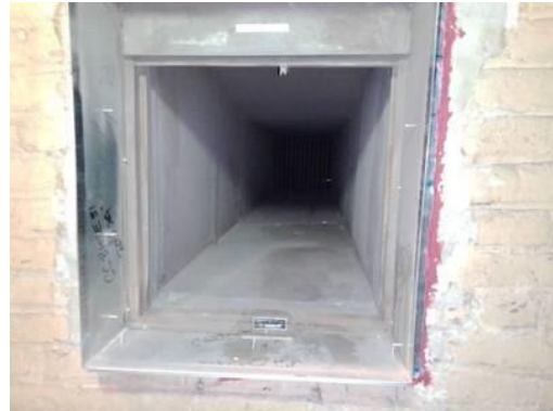
Picture of Damper in Closed Position
