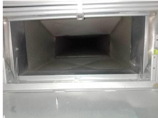
Picture of Damper in Closed Position
