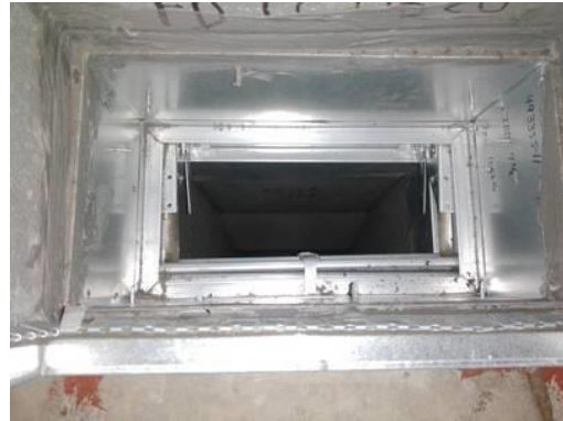
Picture of Damper in Closed Position
