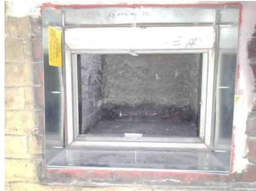
Picture of Damper in Closed Position
