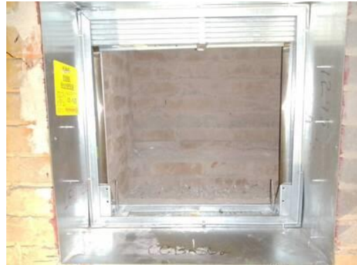
Picture of Damper in Closed Position
