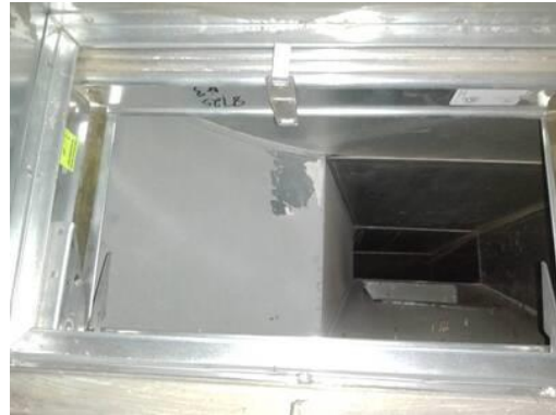
Picture of Damper in Closed Position
