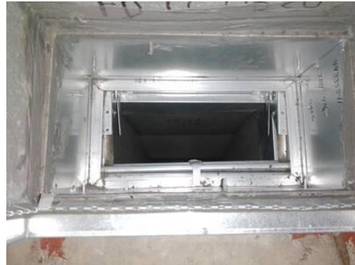
Picture of Damper in Closed Position
