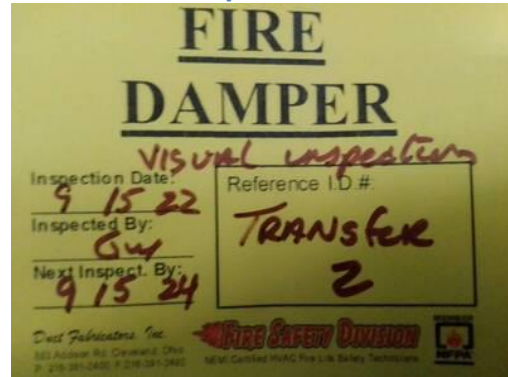
Picture of Damper I.D. Label
