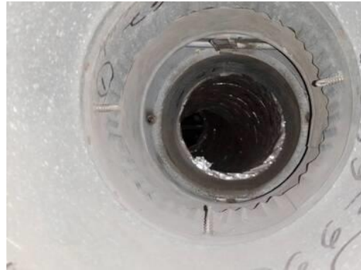
Picture of Damper in Closed Position
