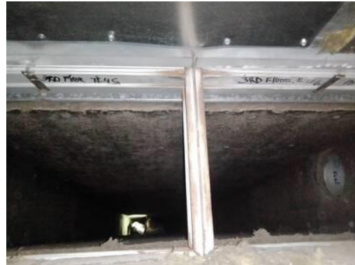
Picture of Damper in Closed Position
