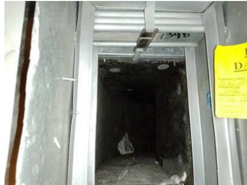
Picture of Damper in Closed Position
