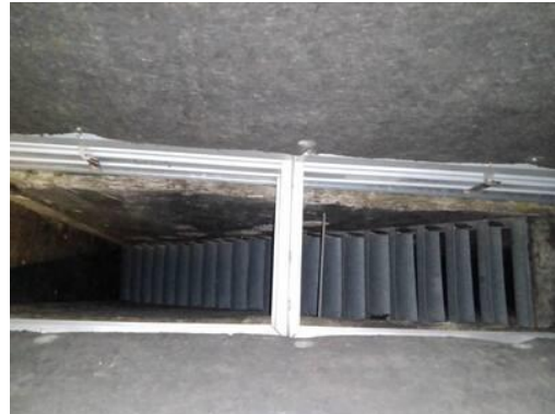
Picture of Damper in Closed Position
