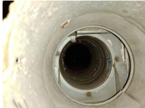
Picture of Damper in Closed Position
