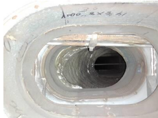
Picture of Damper in Closed Position
