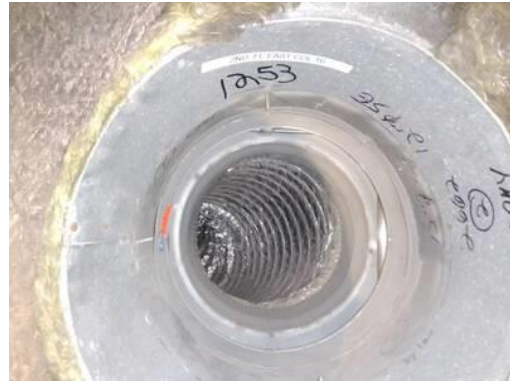
Picture of Damper in Closed Position
