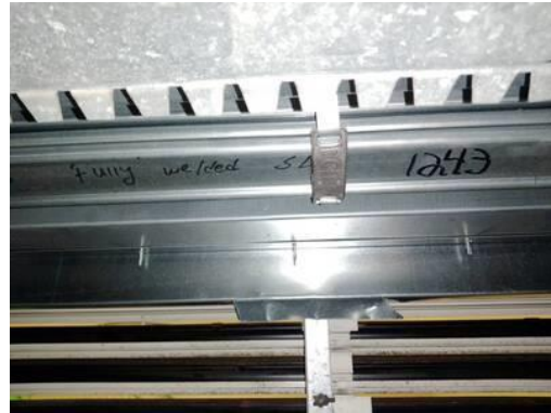
Picture of Damper in Closed Position
