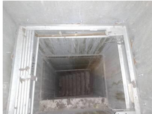
Picture of Damper in Closed Position
