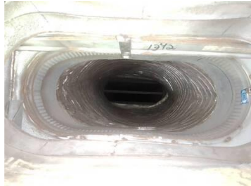
Picture of Damper in Closed Position
