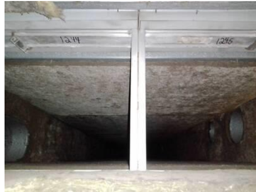
Picture of Damper in Closed Position
