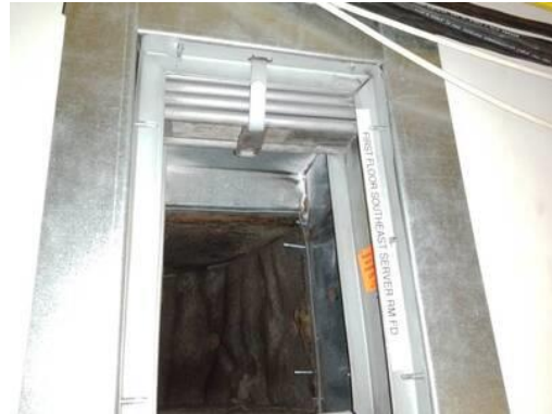
Picture of Damper in Closed Position
