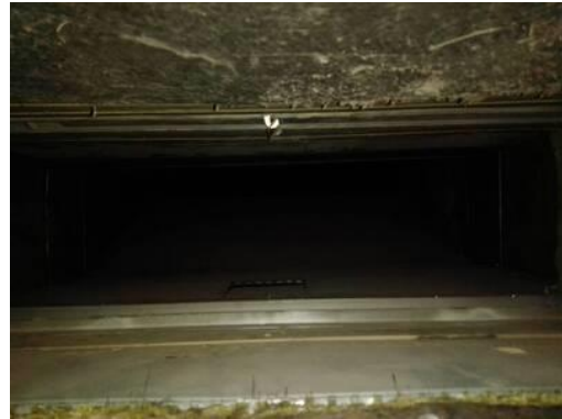
Picture of Damper in Closed Position
