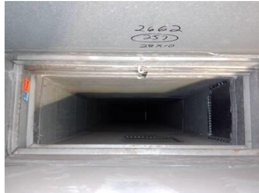
Picture of Damper in Closed Position
