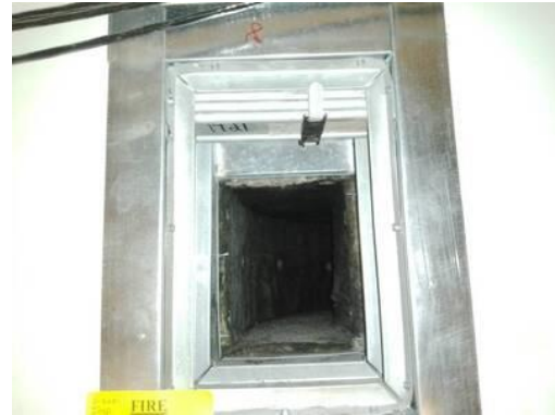
Picture of Damper in Closed Position
