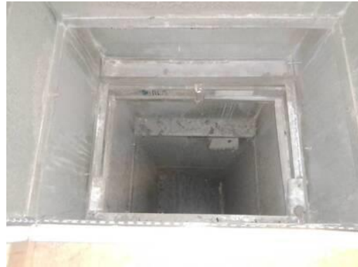
Picture of Damper in Closed Position
