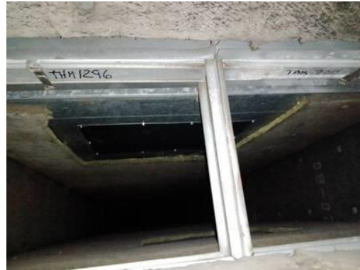
Picture of Damper in Closed Position
