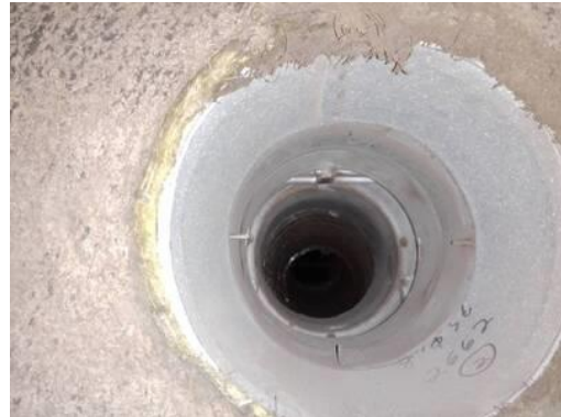
Picture of Damper in Closed Position
