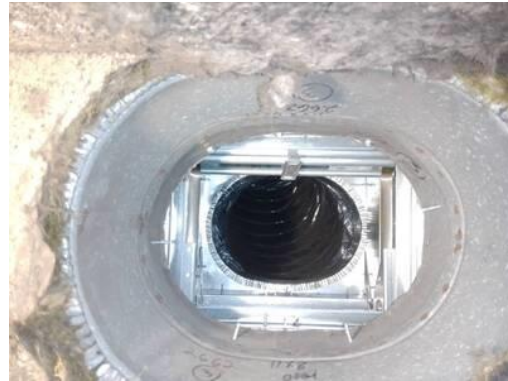
Picture of Damper in Closed Position
