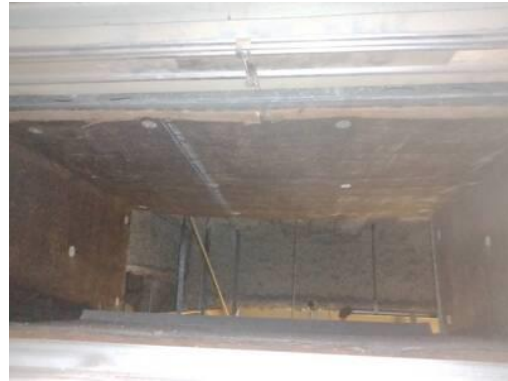
Picture of Damper in Closed Position
