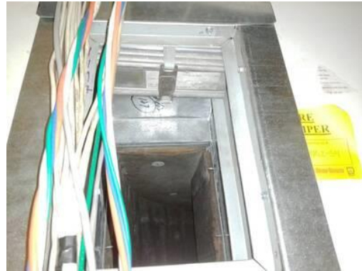
Picture of Damper in Closed Position
