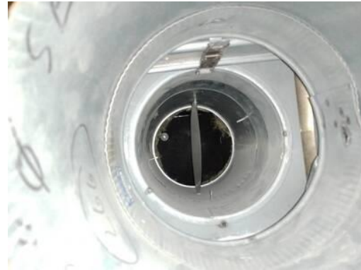
Picture of Damper in Closed Position
