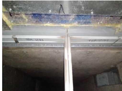
Picture of Damper in Closed Position
