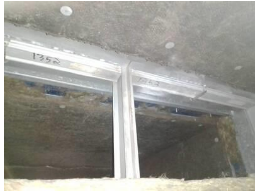
Picture of Damper in Closed Position
