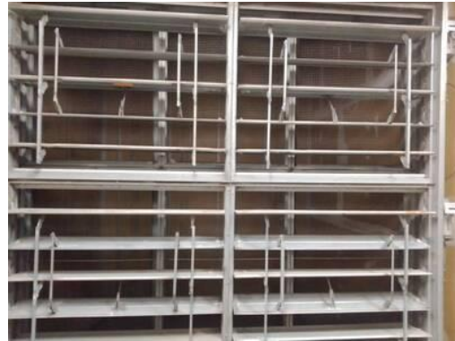
Picture of Damper in Closed Position
