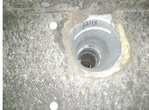
Interior Picture of Damper
