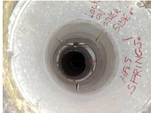
Picture of Damper in Closed Position
