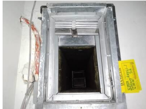
Picture of Damper in Closed Position
