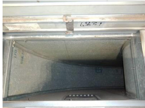
Picture of Damper in Closed Position
