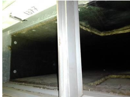
Picture of Damper in Closed Position
