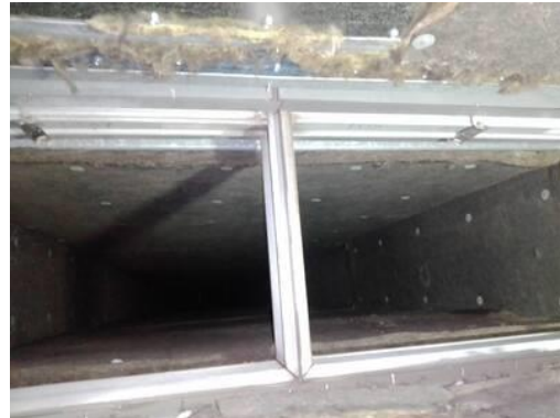
Picture of Damper in Closed Position
