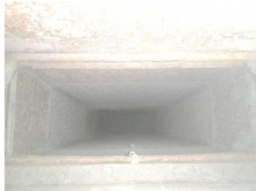
Picture of Damper in Closed Position
