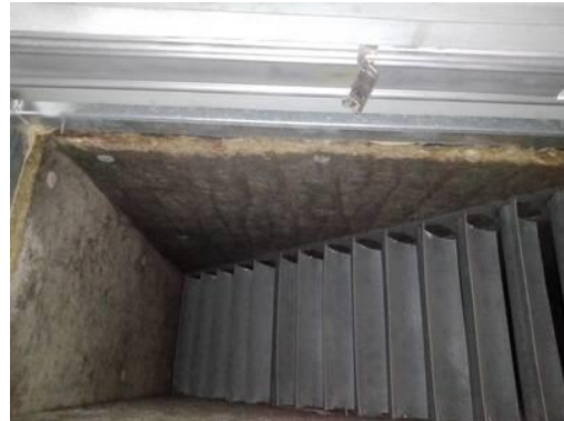
Picture of Damper in Closed Position
