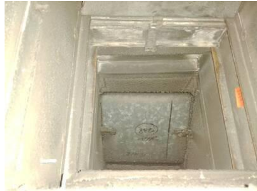
Picture of Damper in Closed Position
