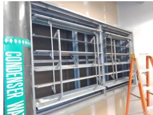
Picture of Damper in Closed Position
