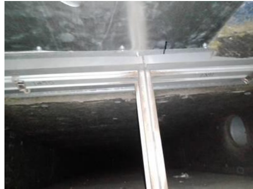
Picture of Damper in Closed Position
