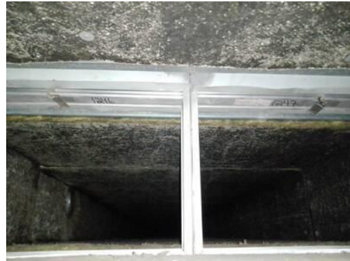
Picture of Damper in Closed Position
