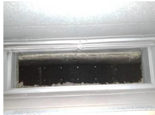
Picture of Damper in Closed Position
