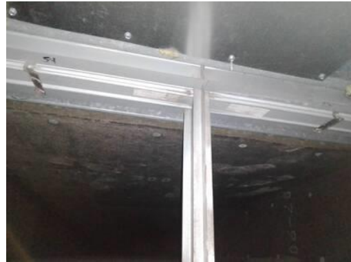
Picture of Damper in Closed Position
