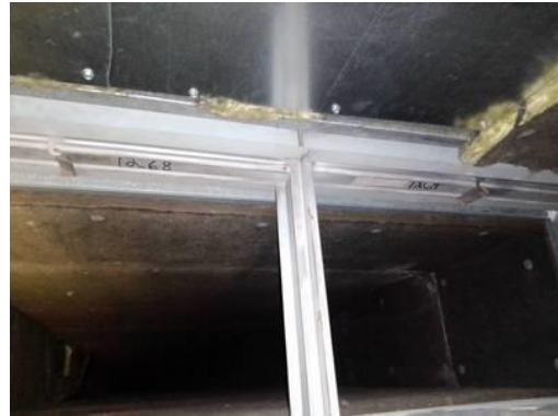
Picture of Damper in Closed Position
