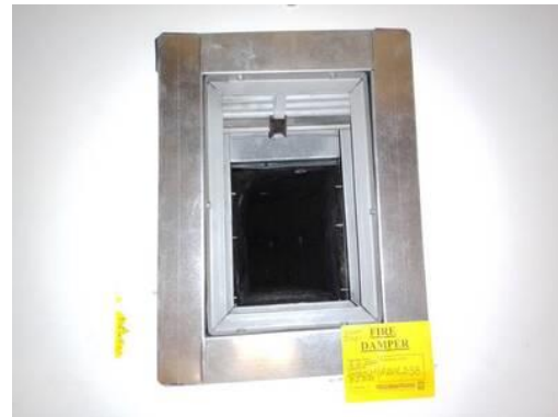
Picture of Damper in Closed Position
