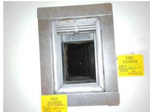
Picture of Damper in Closed Position
