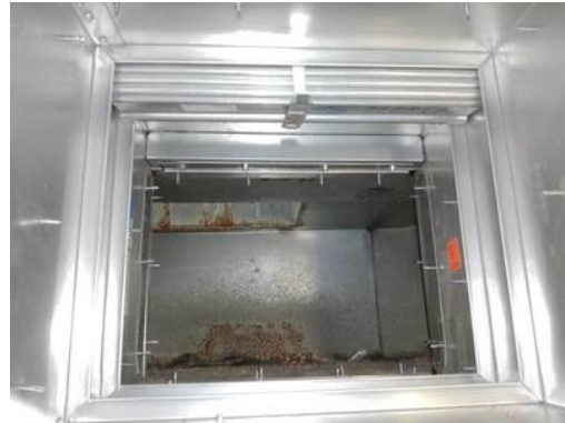
Picture of Damper in Closed Position
