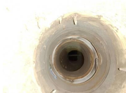
Picture of Damper in Closed Position
