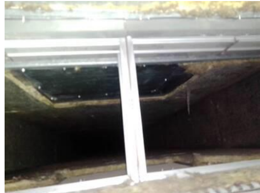
Picture of Damper in Closed Position
