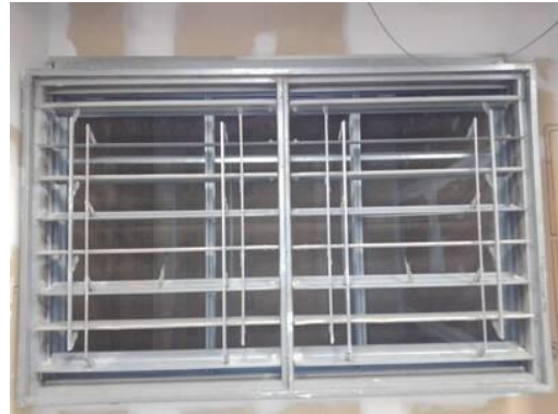
Picture of Damper in Closed Position
