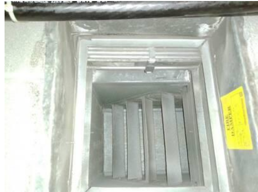
Picture of Damper in Closed Position
