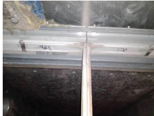
Picture of Damper in Closed Position
