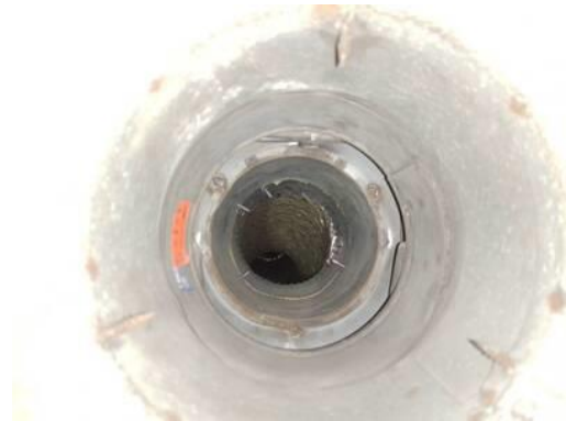
Picture of Damper in Closed Position
