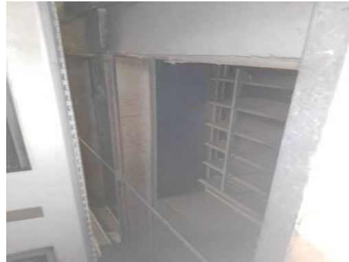
Picture of Damper in Closed Position
