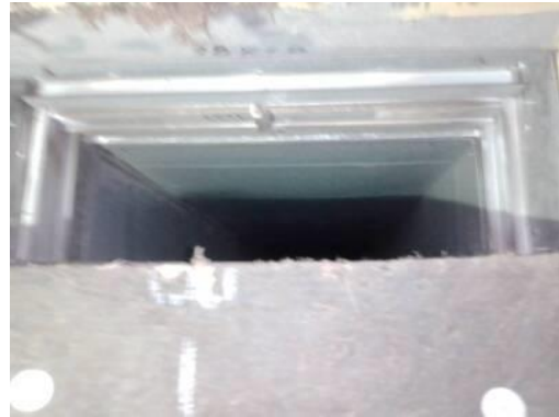
Picture of Damper in Closed Position
