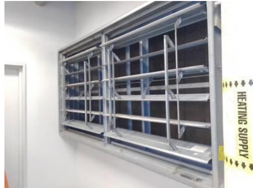
Picture of Damper in Closed Position
