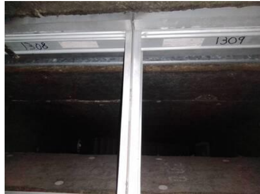
Picture of Damper in Closed Position
