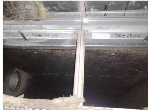
Picture of Damper in Closed Position
