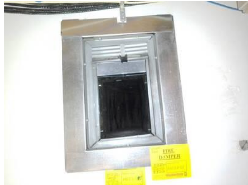
Picture of Damper in Closed Position
