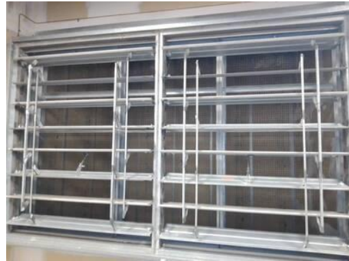
Picture of Damper in Closed Position
