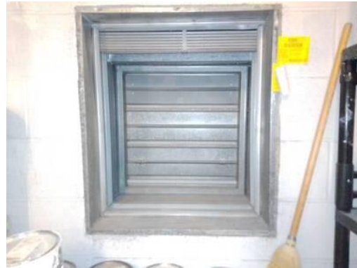
Picture of Damper in Closed Position
