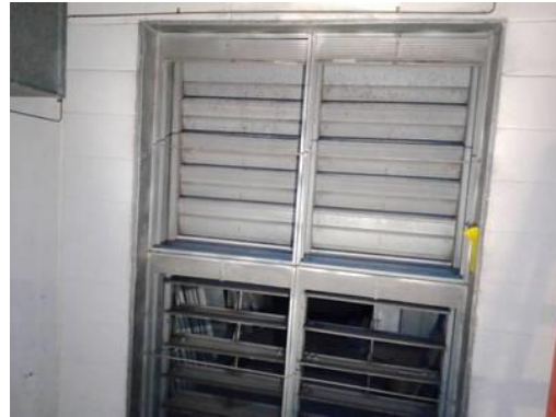
Picture of Damper in Closed Position
