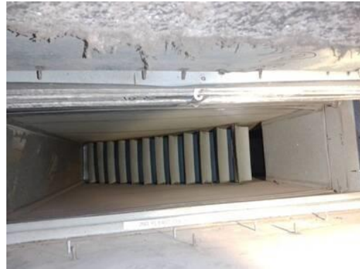
Picture of Damper in Closed Position
