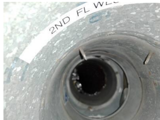
Picture of Damper in Closed Position
