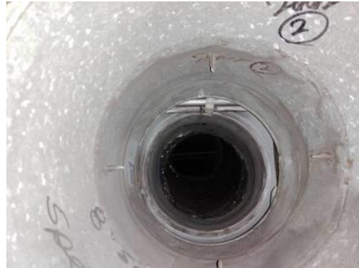
Picture of Damper in Closed Position
