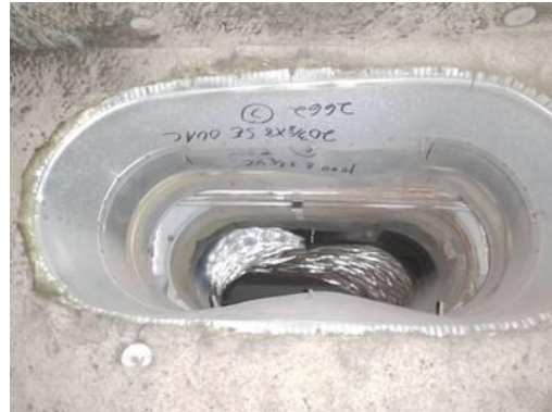
Picture of Damper in Closed Position
