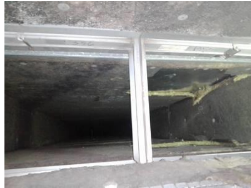
Picture of Damper in Closed Position
