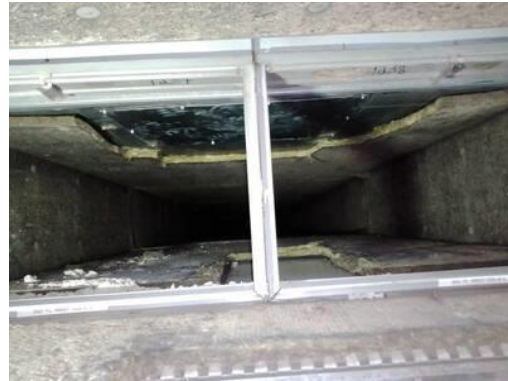
Picture of Damper in Closed Position
