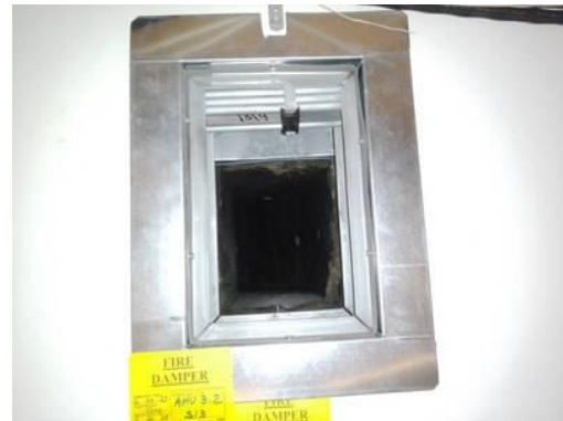
Picture of Damper in Closed Position
