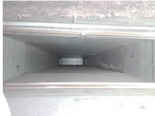
Picture of Damper in Closed Position
