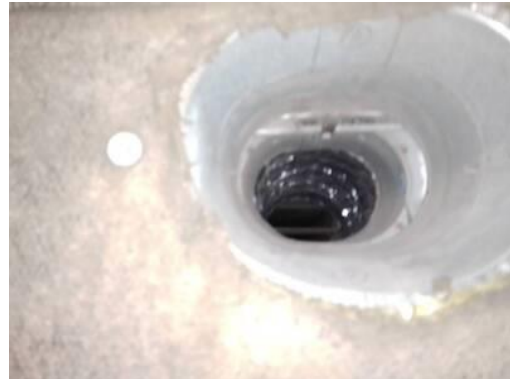
Picture of Damper in Closed Position
