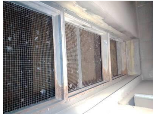
Picture of Damper in Closed Position
