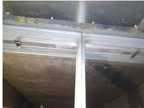
Picture of Damper in Closed Position
