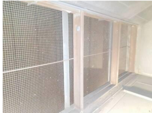
Picture of Damper in Closed Position
