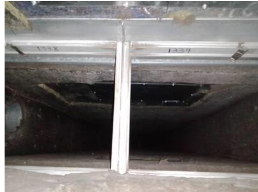
Picture of Damper in Closed Position
