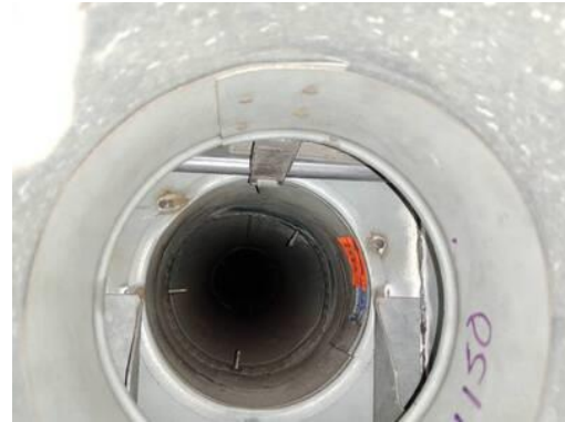
Picture of Damper in Closed Position
