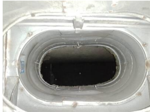
Picture of Damper in Closed Position
