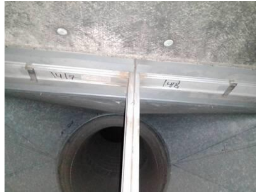
Picture of Damper in Closed Position
