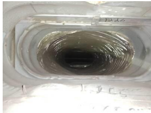
Picture of Damper in Closed Position
