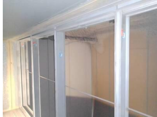
Picture of Damper in Closed Position
