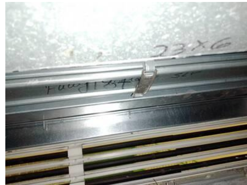
Picture of Damper in Closed Position
