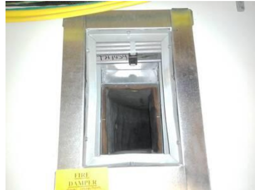
Picture of Damper in Closed Position
