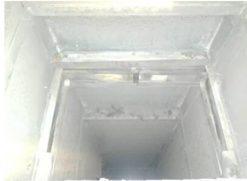
Picture of Damper in Closed Position
