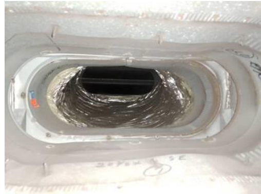
Picture of Damper in Closed Position
