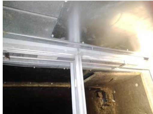
Picture of Damper in Closed Position
