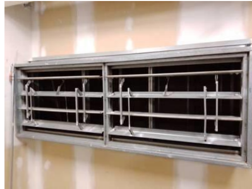
Picture of Damper in Closed Position
