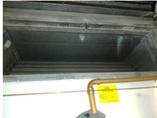
Picture of Damper in Closed Position
