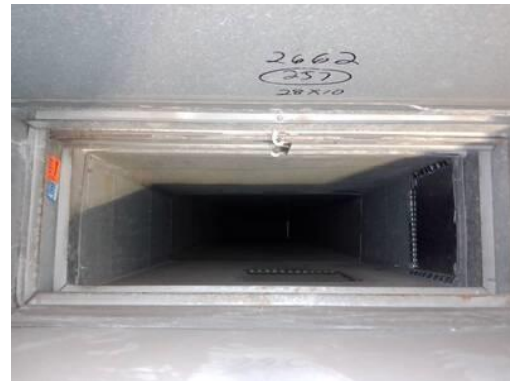
Picture of Damper in Closed Position
