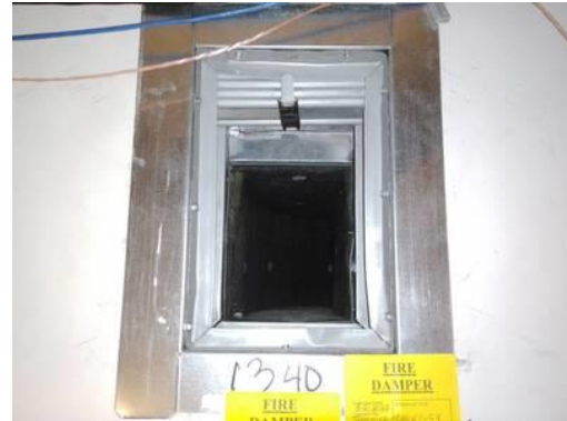
Picture of Damper in Closed Position
