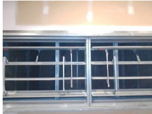
Picture of Damper in Closed Position
