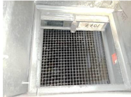
Picture of Damper in Closed Position
