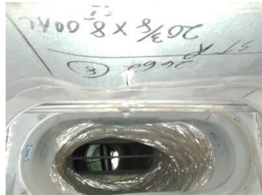
Picture of Damper in Closed Position
