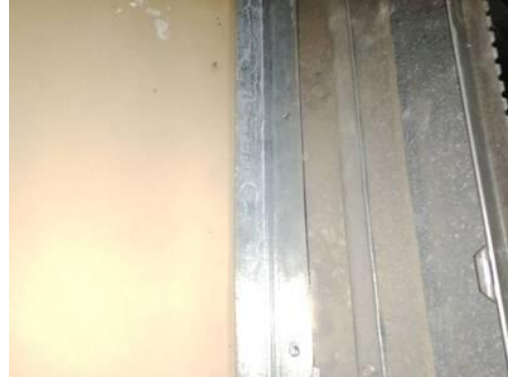
Interior Picture of Damper
