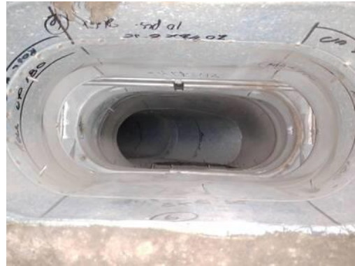
Picture of Damper in Closed Position
