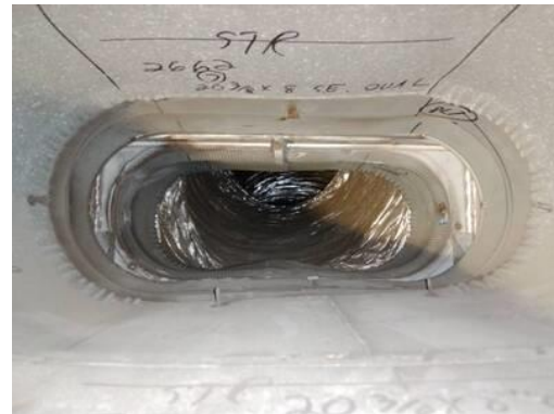
Picture of Damper in Closed Position
