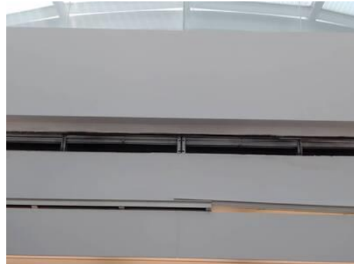
Picture of Damper in Closed Position
