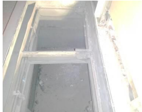
Picture of Damper in Closed Position
