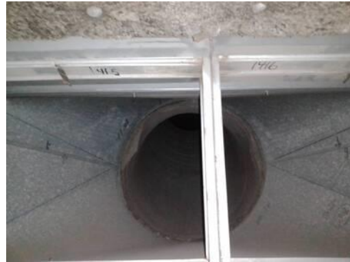
Picture of Damper in Closed Position
