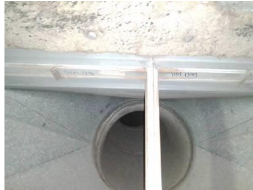
Picture of Damper in Closed Position
