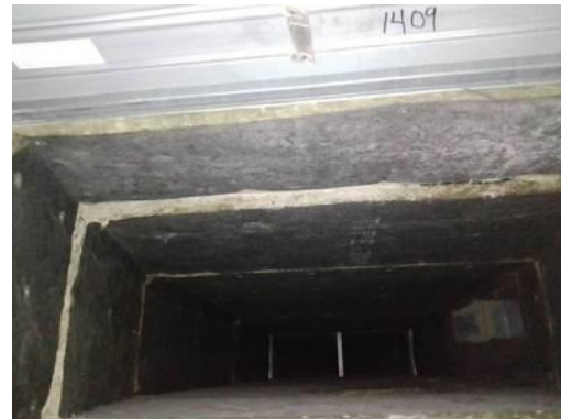
Picture of Damper in Closed Position
