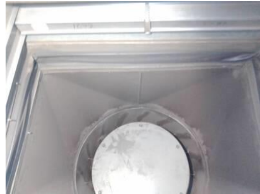
Picture of Damper in Closed Position
