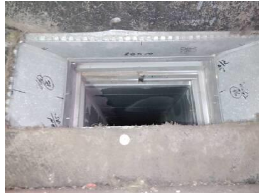
Picture of Damper in Closed Position
