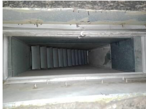
Picture of Damper in Closed Position
