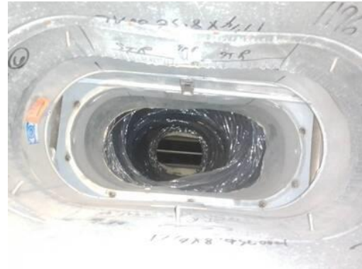
Picture of Damper in Closed Position
