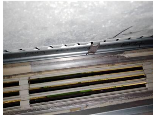
Picture of Damper in Closed Position
