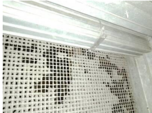
Picture of Damper in Closed Position
