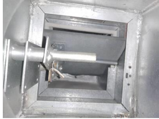
Picture of Damper in Closed Position
