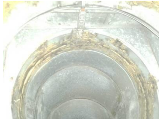
Picture of Damper in Closed Position
