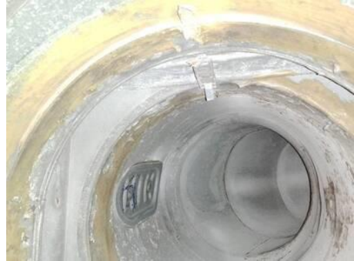
Picture of Damper in Closed Position
