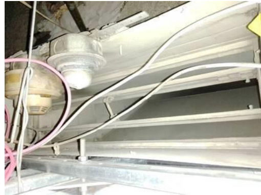
Picture of Damper in Closed Position
