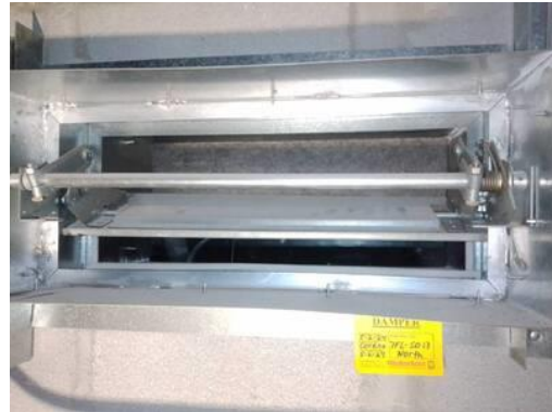
Picture of Damper in Closed Position
