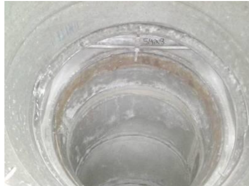
Picture of Damper in Closed Position
