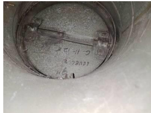
Picture of Damper I.D. Label
