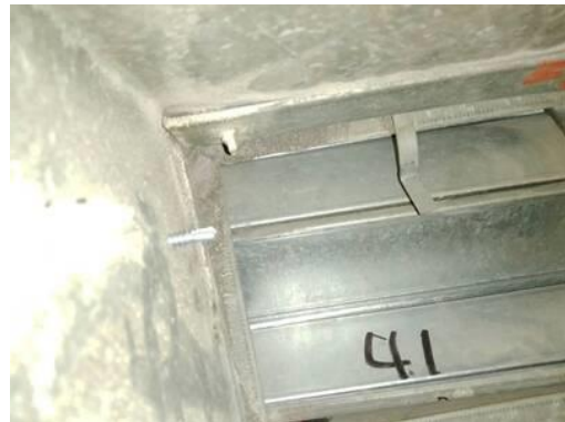
Picture of Damper I.D. Label
