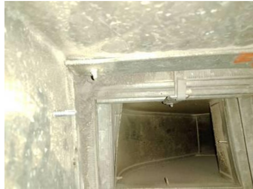
Picture of Damper in Closed Position
