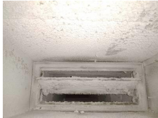
Picture of Damper in Closed Position
