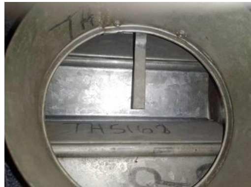
Picture of Damper I.D. Label
