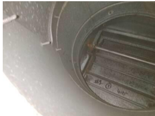
Picture of Damper I.D. Label
