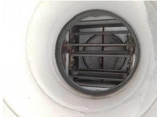
Picture of Damper in Closed Position
