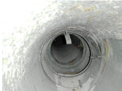
Picture of Damper in Closed Position
