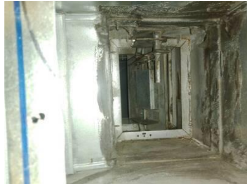
Picture of Damper in Closed Position
