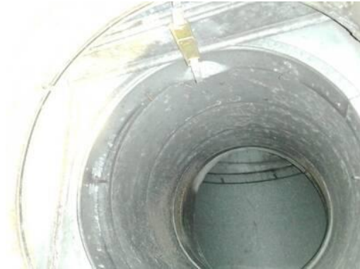
Picture of Damper in Closed Position
