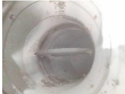
Picture of Damper in Closed Position
