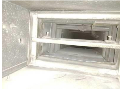
Picture of Damper in Closed Position
