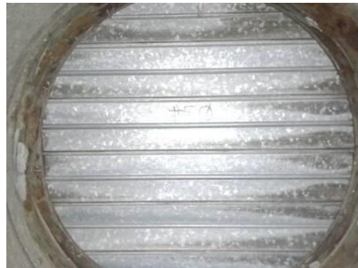
Picture of Damper I.D. Label
