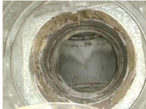
Picture of Damper in Closed Position
