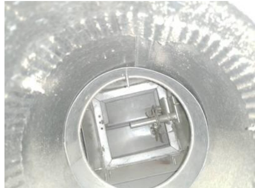
Picture of Damper I.D. Label
