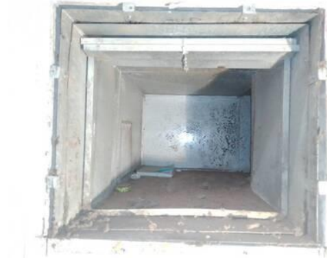
Picture of Damper in Closed Position
