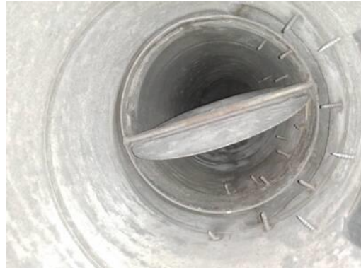
Picture of Damper in Closed Position
