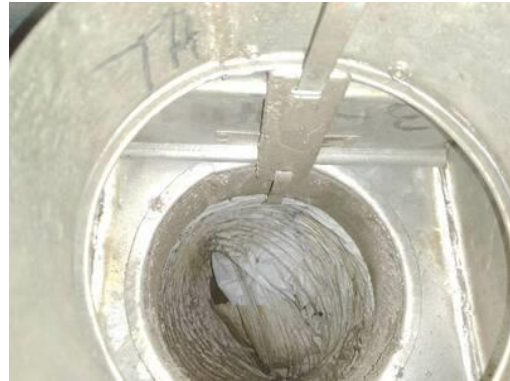
Picture of Damper in Closed Position
