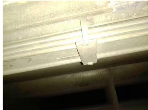
Picture of Damper in Closed Position
