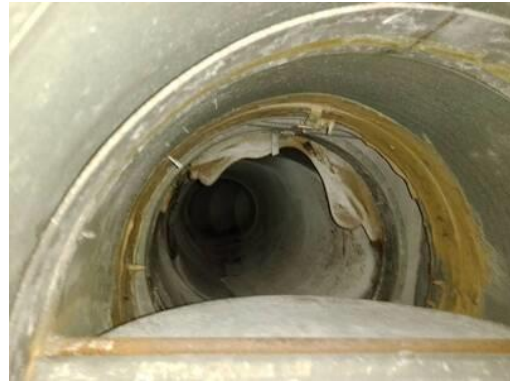
Picture of Damper in Closed Position
