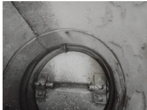
Picture of Damper I.D. Label
