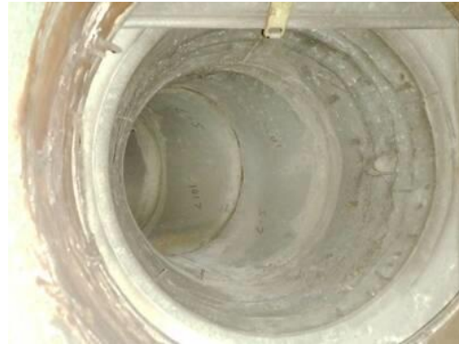
Picture of Damper in Closed Position
