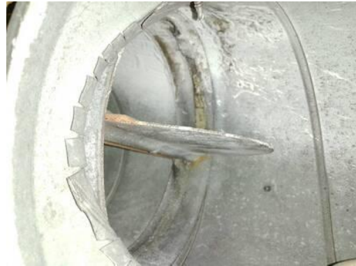
Picture of Damper in Closed Position
