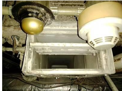
Picture of Damper in Closed Position
