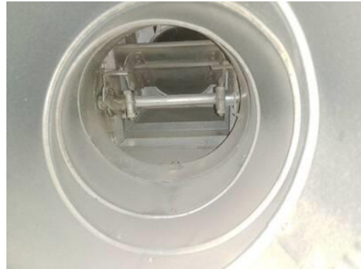
Picture of Damper in Closed Position
