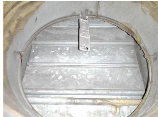
Picture of Damper I.D. Label
