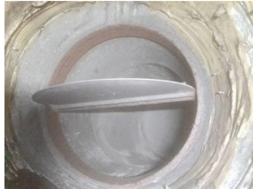
Picture of Damper in Closed Position
