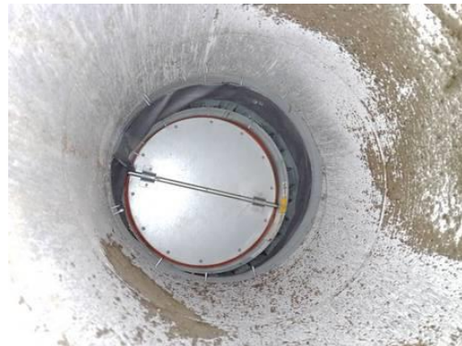
Picture of Damper I.D. Label
