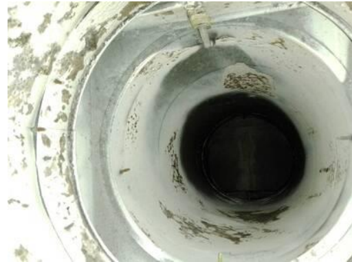
Picture of Damper in Closed Position
