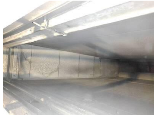
Picture of Damper in Closed Position
