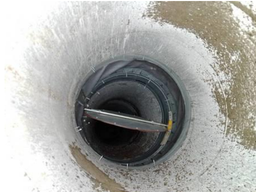
Picture of Damper in Closed Position
