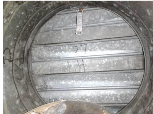
Picture of Damper I.D. Label
