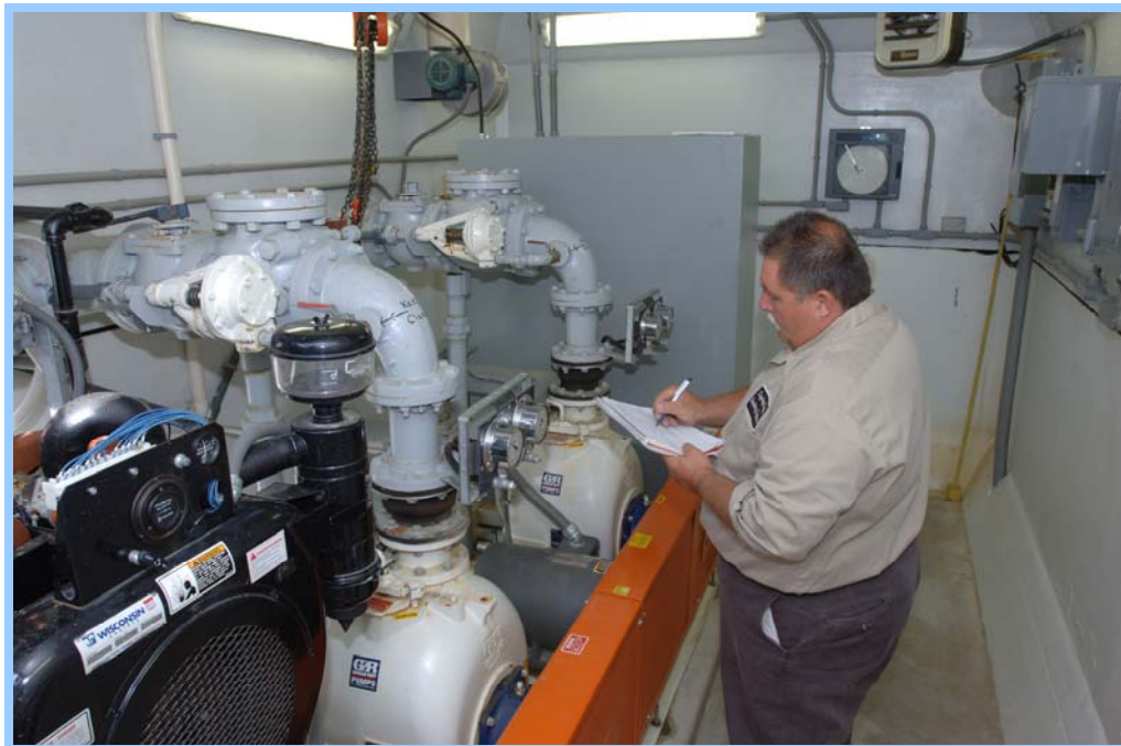
* Valley Ranch Pump Station
