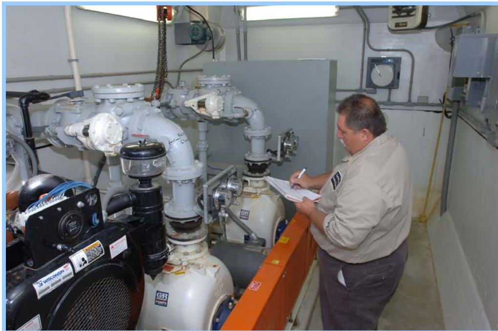
* Valley Ranch Pump Station
