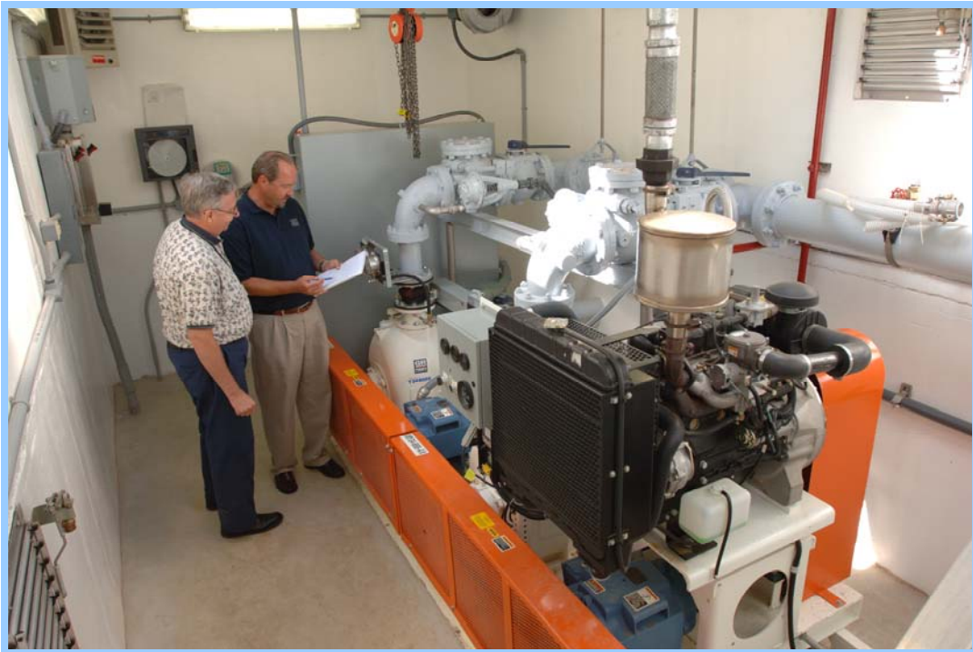
* Brainard Pump Station
