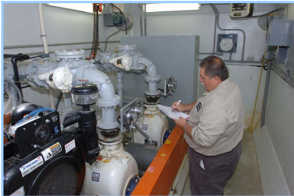
* Valley Ranch Pump Station
