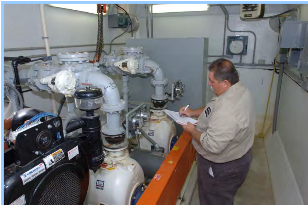
* Valley Ranch Pump Station
