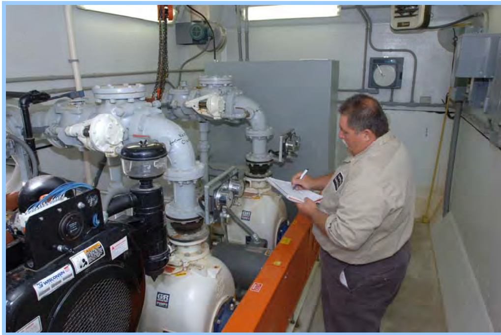
* Valley Ranch Pump Station
