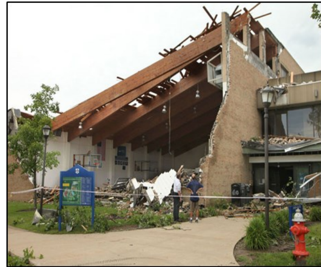
Tornado damage at Ursuline College, July 20, 2013
