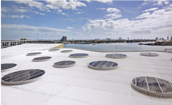
Solar canopy at NRG Miami Heat Arena in Miami. Photo by Moris Moreno.
