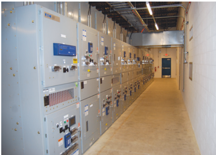
Block building containing switchgear
