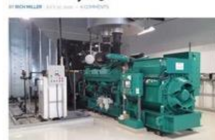
A backup generator at a Microsoft data center in Oregon. (Photo: Rich Miller)
