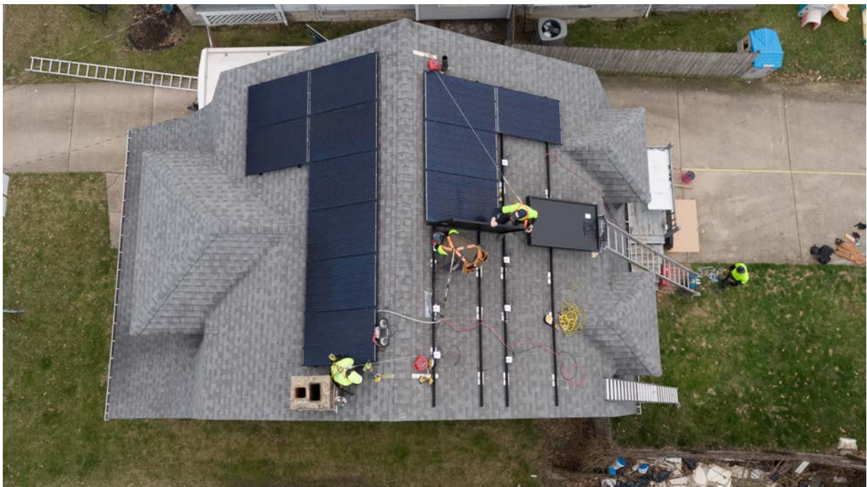
Solar panels installed on a home in Lakewood.
